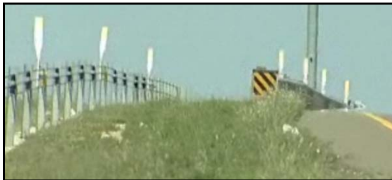
Figure 2-38. Picture Showing Special Extended Delineators.
