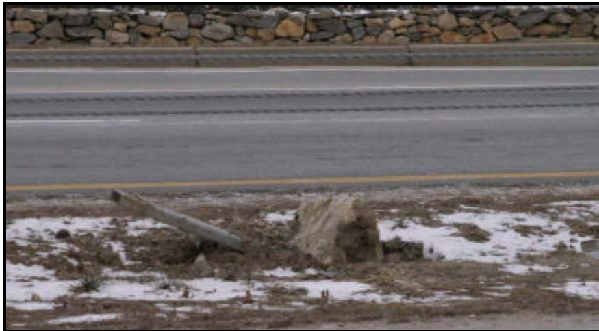
Figure 2-35. Example Photograph of Dislodged Anchor Terminal in Rhode Island (60).
