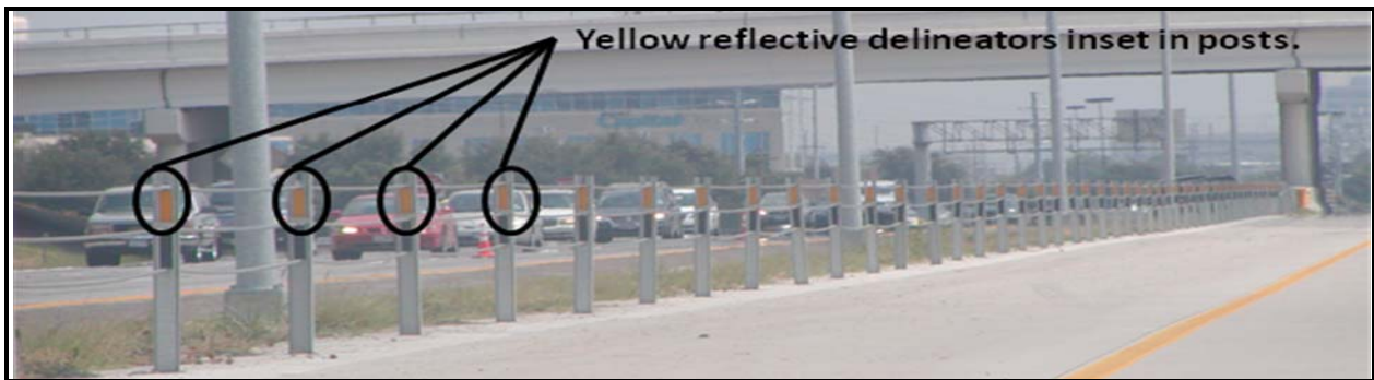
Figure 2-37. Picture Showing Delineators Inset in Cable Barrier Posts.
