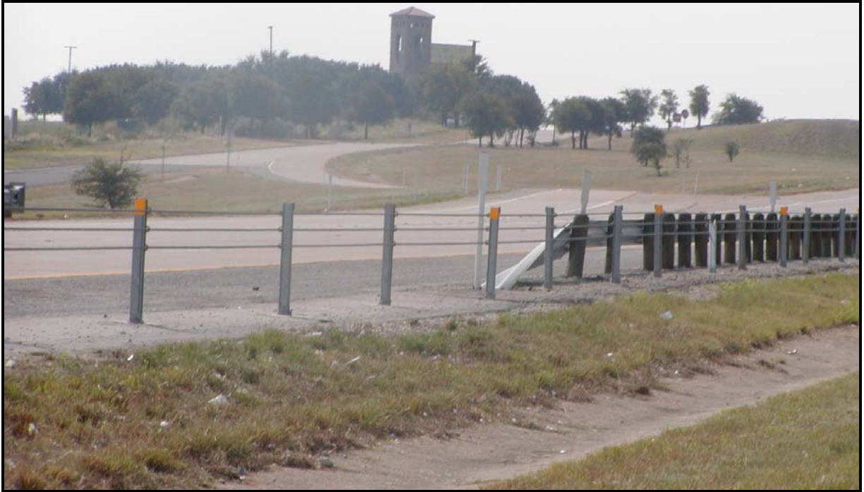
Figure 3-4. Example to Avoid: Inadequate Spacing between Cable Barrier and MBGF.
