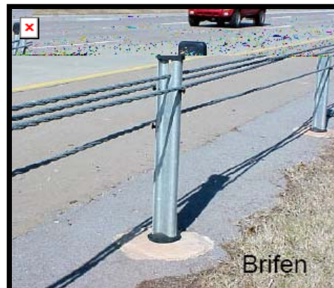
Figure 2-6. Brifen Wire Rope Safety Fence.
