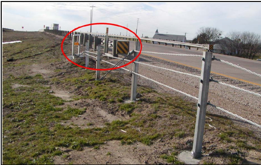
Figure 3-5. Anchor Terminals Too Close to Guardrail End Treatments Can Cause Problems.
