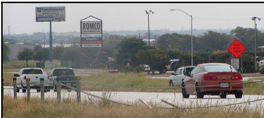
Figure 4-15. IH 820 Northwest Loop in Fort Worth – Damage Is Not Repaired.
