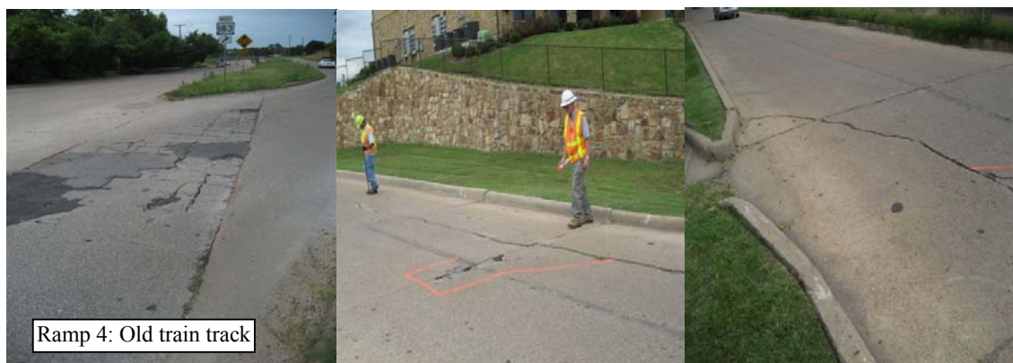
Figure 22. Observed Distresses on the Ramps, Pumphrey Drive, FTW.
