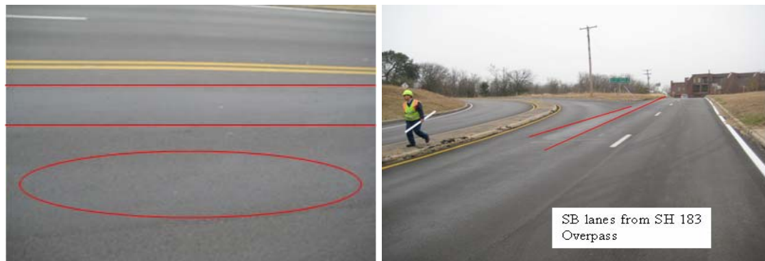
Figure 26. Potential Spots for Flushing/Bleeding (Mostly on the Latex Surface).
