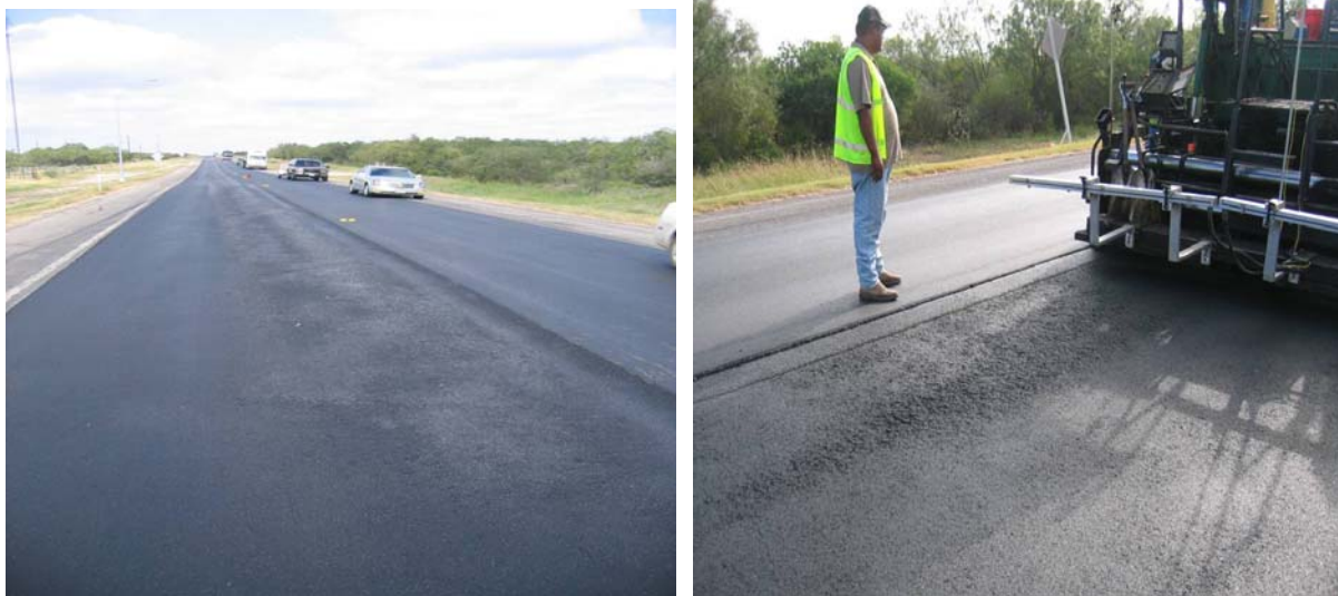
Figure 40. Placement Problems with the CAM on US 90.
