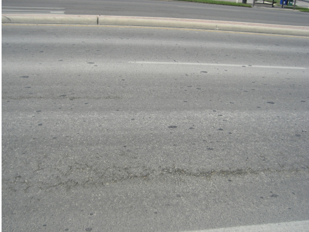
Figure 5.13. Evidence of Cracking Appearing in Both WMA and HMA Sections.
