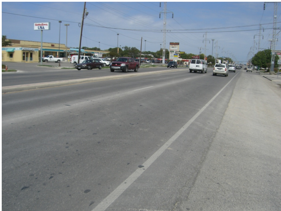
Figure 5.12. San Antonio WMA Section after 3 Years of Service.
