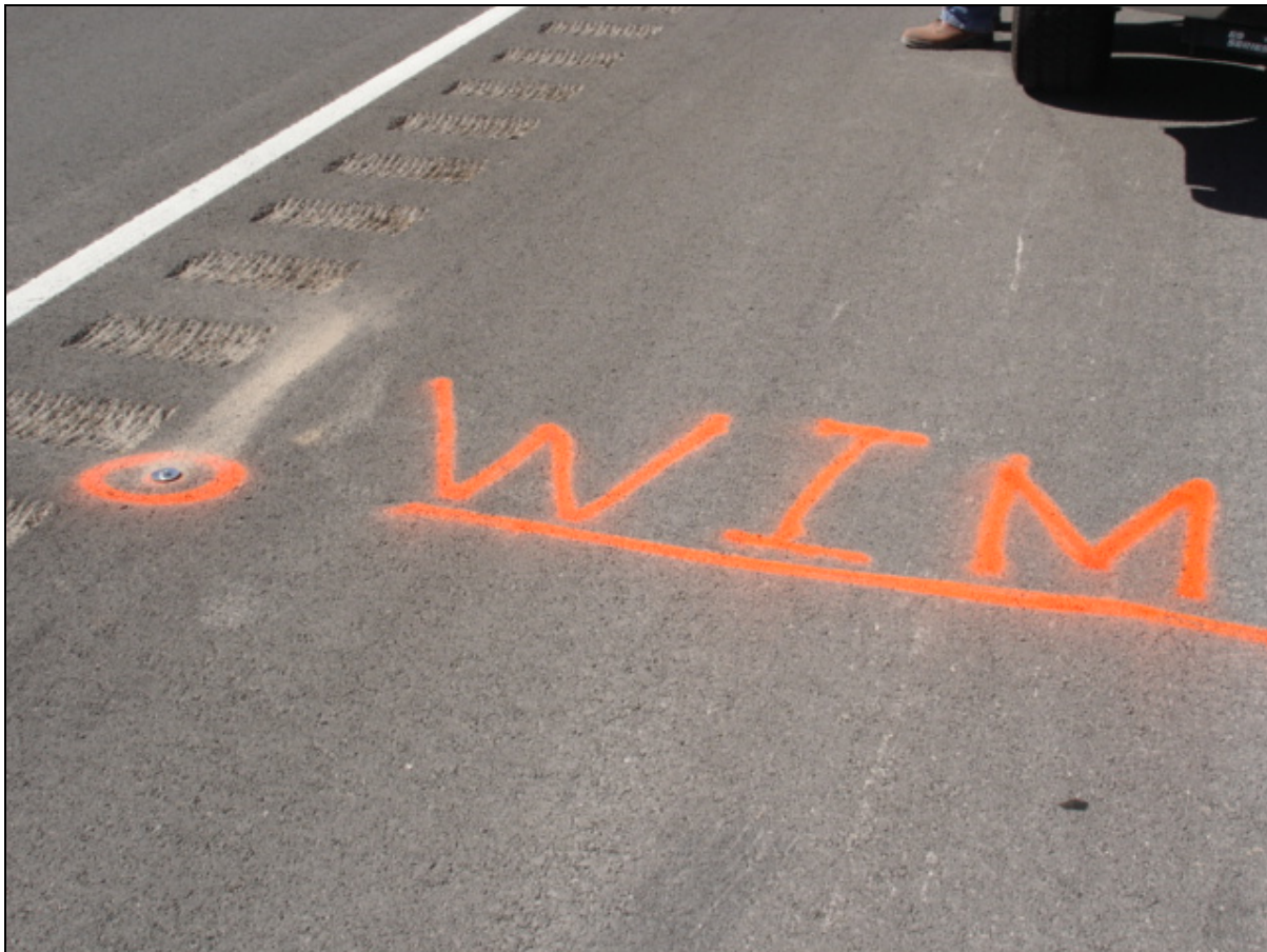
Figure E3. Marker Placed at Proposed Location of WIM Sensors on Westbound Lanes.
