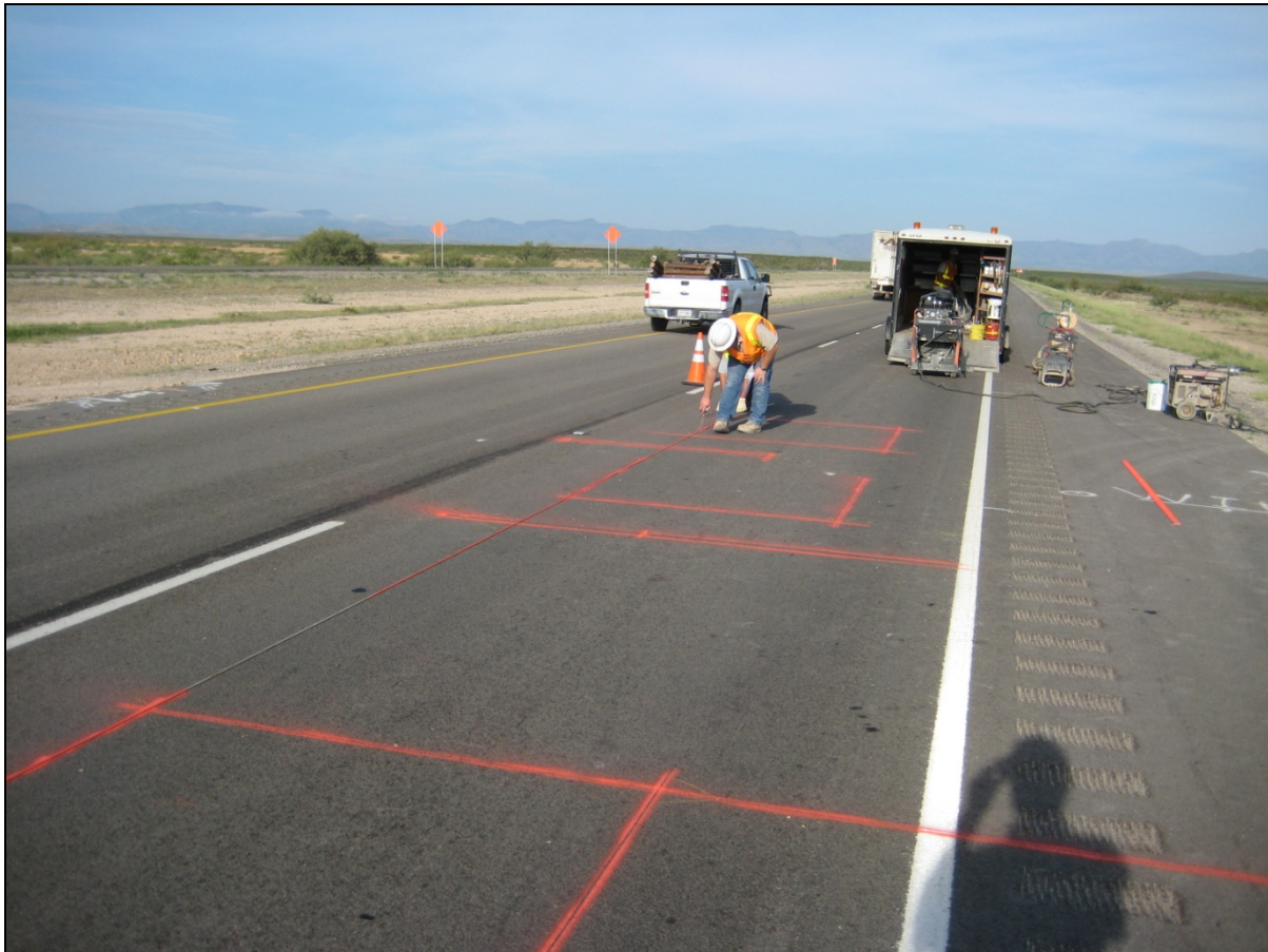
Figure 4.2. Photo of Balmorhea WIM Installation.
