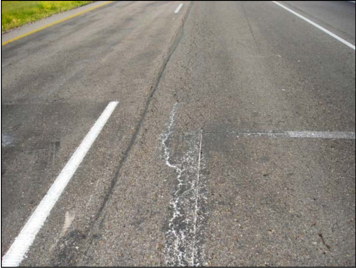
Figure 3.18. Cracking on US77 Northbound Outside Lane (from August 2008 Visit).
