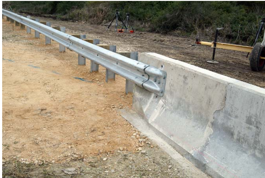
Figure 3-8. Photo of Texas TL-2 Guardrail-to-Concrete Bridge Rail Transition.
