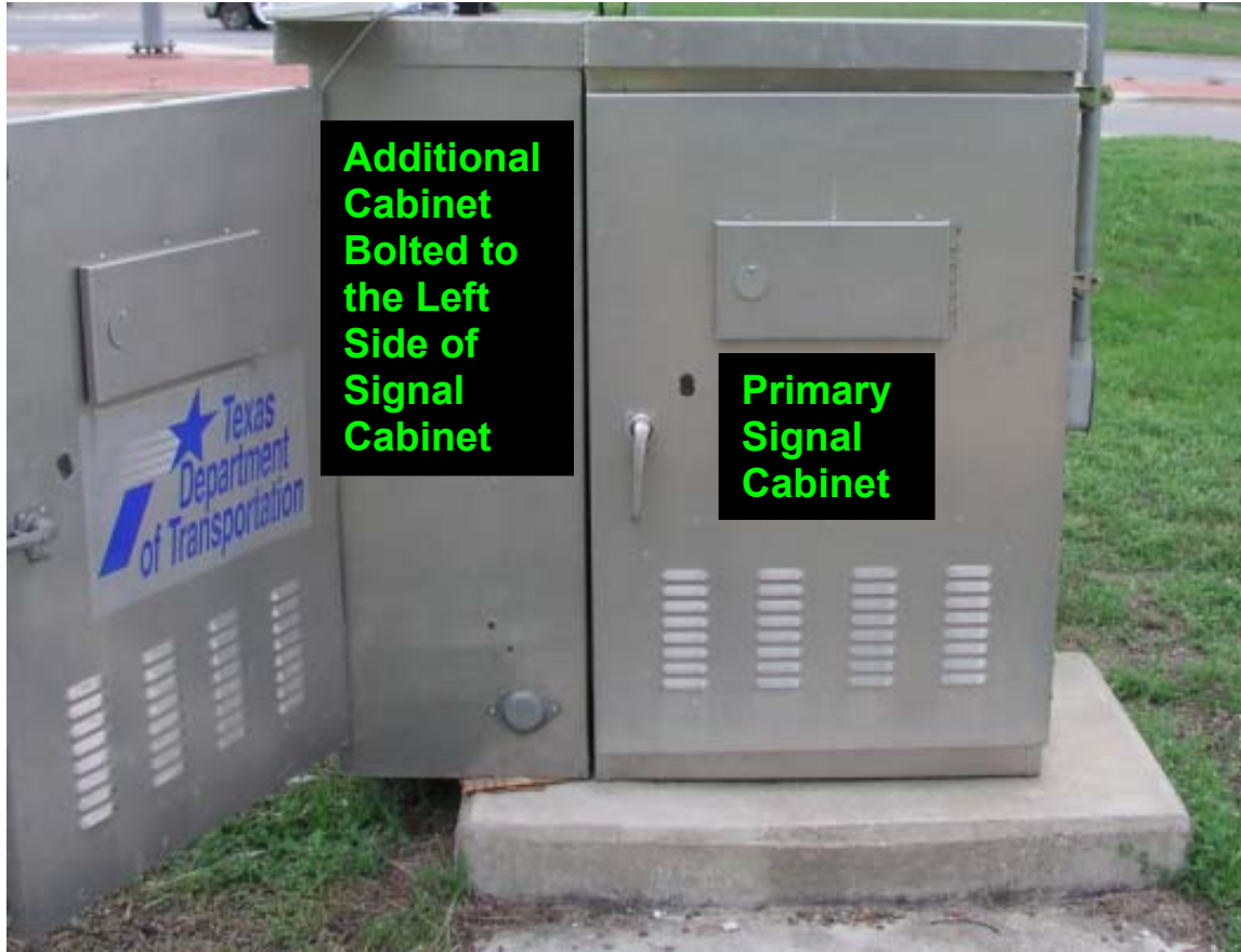
Figure 20. Additional Cabinet Installed for the PIA-2 System.
