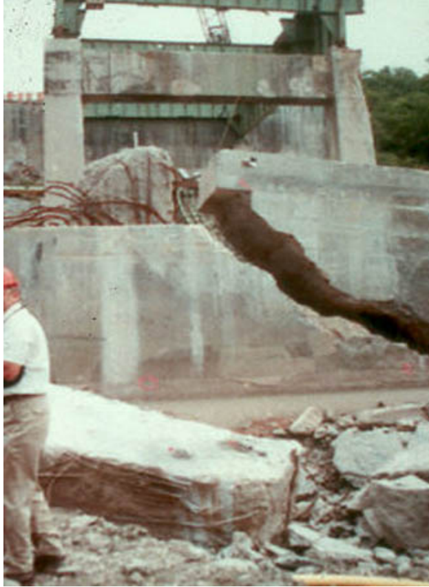
Figure 8-11. Photo of Pier 3 Taken in 1987 after the Failure.
