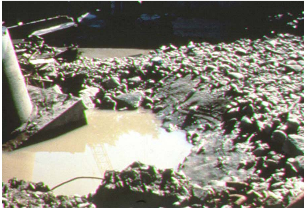
Figure 8-10. Photo of Pier 2 Taken in 1987 after the Failure.
