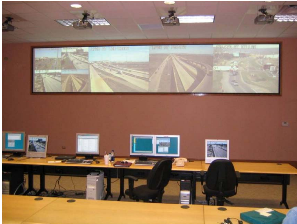
Figure 2-21: Laredo's TMC – STRATIS.
