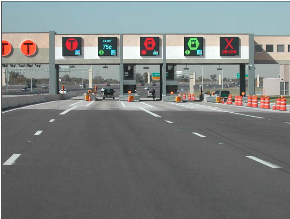
Figure 21. Focus Group Slide 7 Showing Full Plaza with Open-Road Tolling Lanes on Left.
