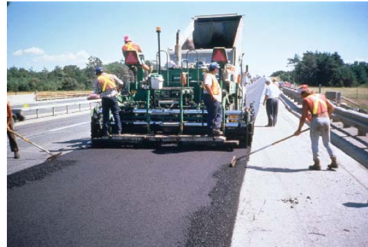
Figure 21. Improper Raking of the Longitudinal Joint (Scherozman 2004)
