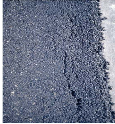
Figure 19. Crack Development in the Mix at the Unsupported Edge of Pavement (Scherozman 2004)
