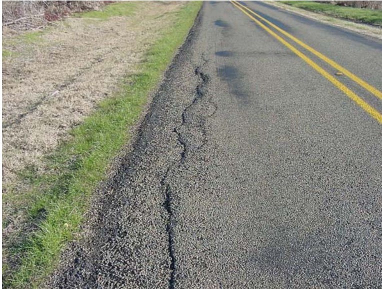
Figure 2: Flexible Pavement Section in Poor Condition
