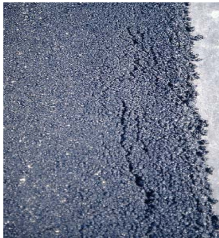
Figure 13. Crack Development in the Mix at the Unsupported Edge of Pavement (Scherozman 2004).
