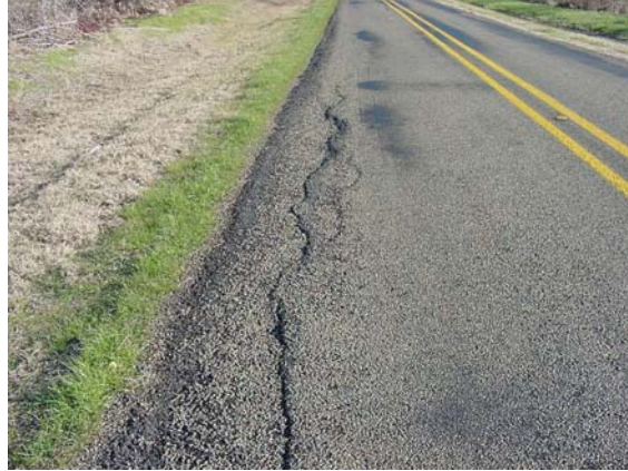
Figure 28. Flexible Pavement Section in Poor Condition.
