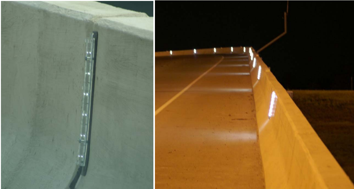
Figure 10. Curve Warning Barrier Markings. (Photo courtesy of TTI)
