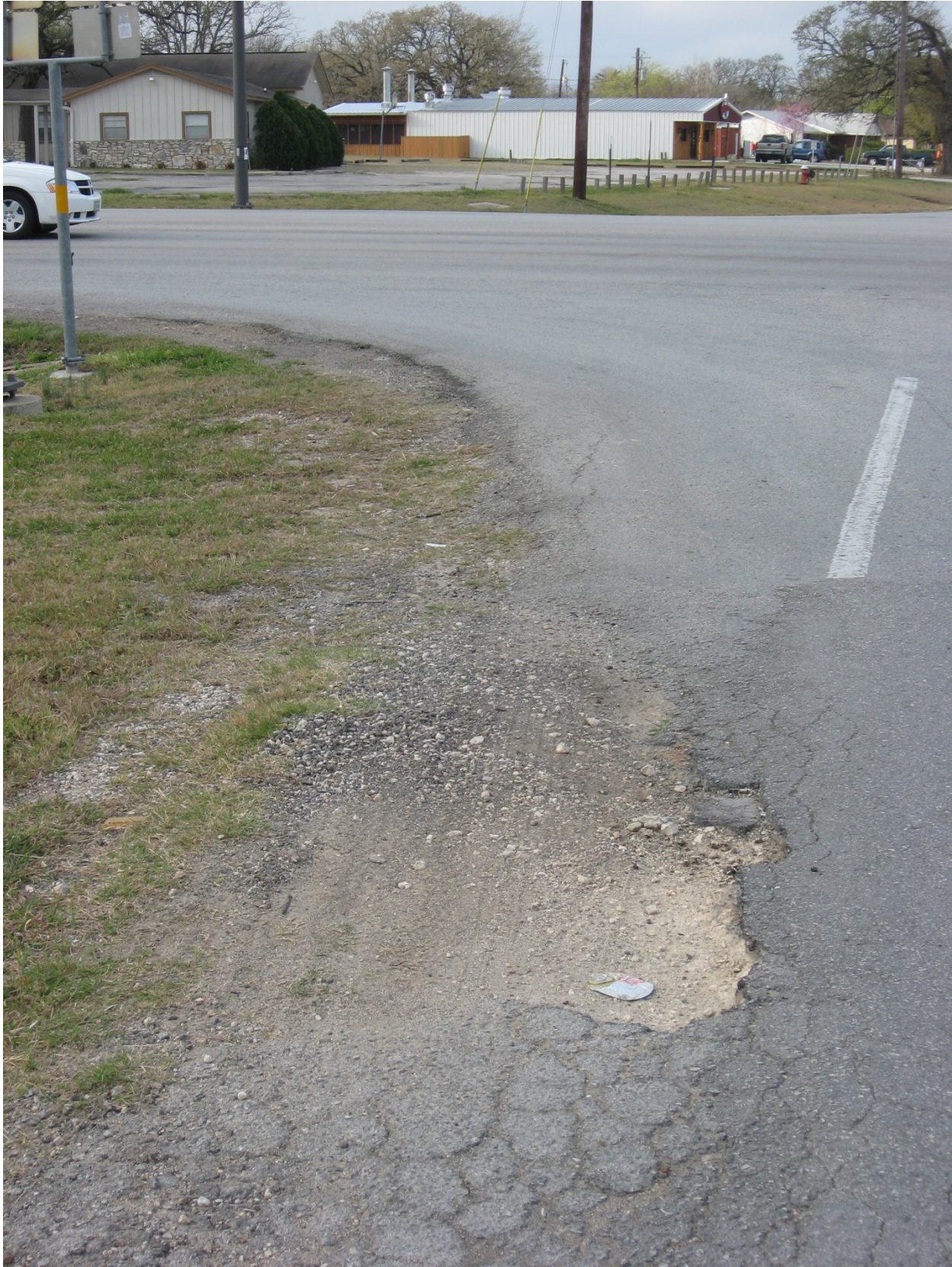
Figure 1. Pavement Damage from Trucks Tracking Off Pavement at a Short Corner Radius.
