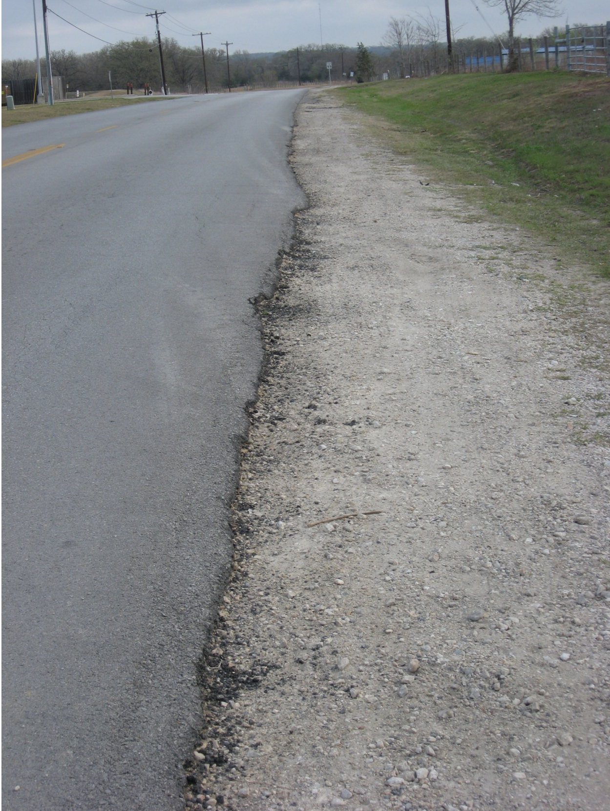
Figure 2. Broken Pavement Edge Where Truck Tires Have Tracked over the Edge.
