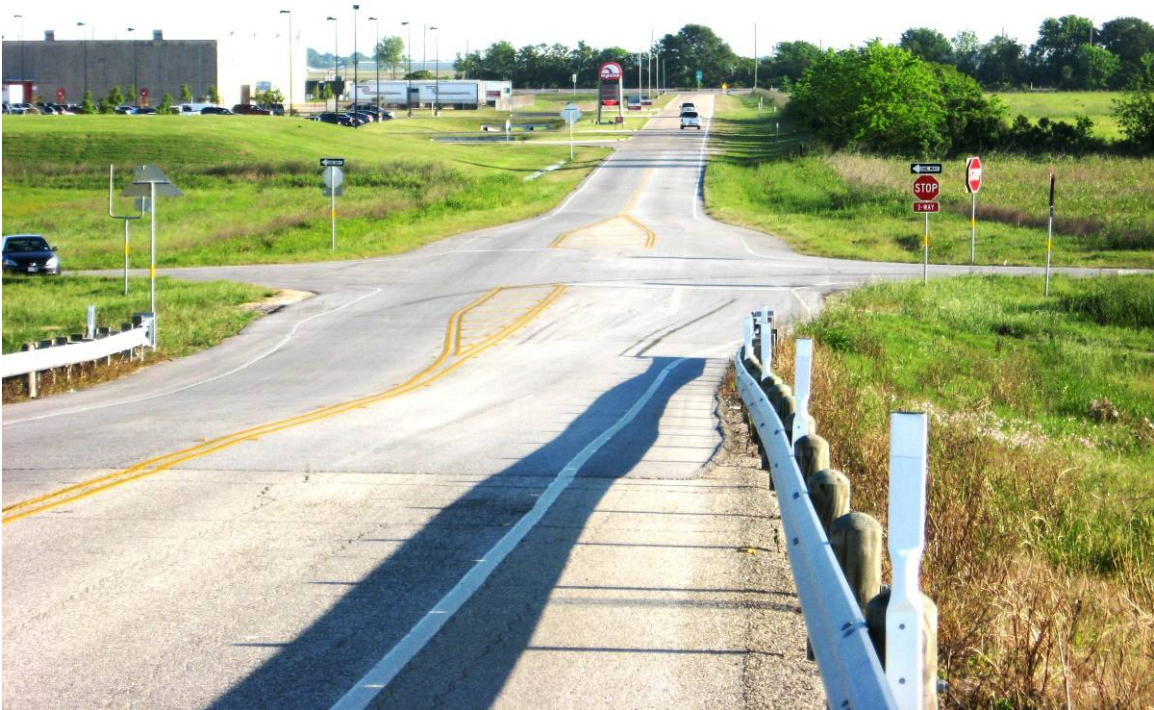
Figure 7. Igloo Repaved Igloo Road with Concrete Adjacent to DC Property to Protect against Deterioration due to Tire Scraping in Tight Turns.
