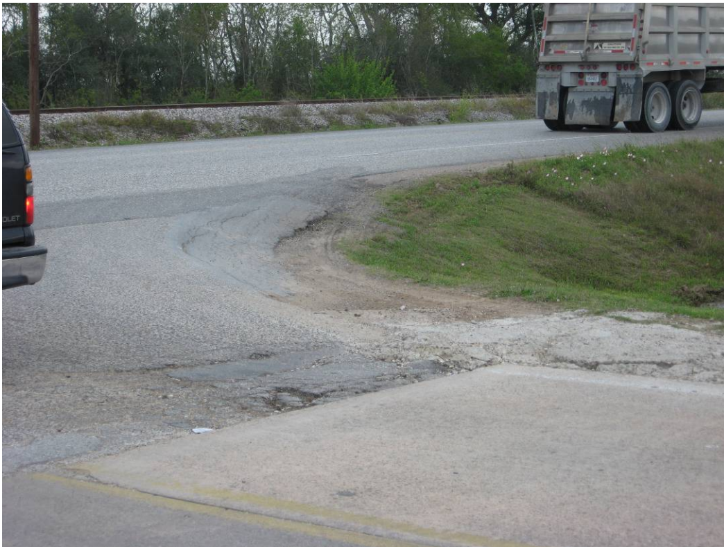
Figure 5. Insufficient Turning Radius and Pavement Failure with Some Patching, Igloo Road and US 90.
