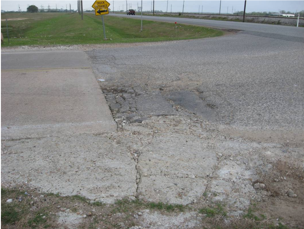
Figure 6. Pavement Failure at Igloo Road and US 90.
