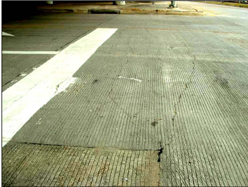
Figure 3-2 Restraint Cracking from Drainage Inlet Box.
