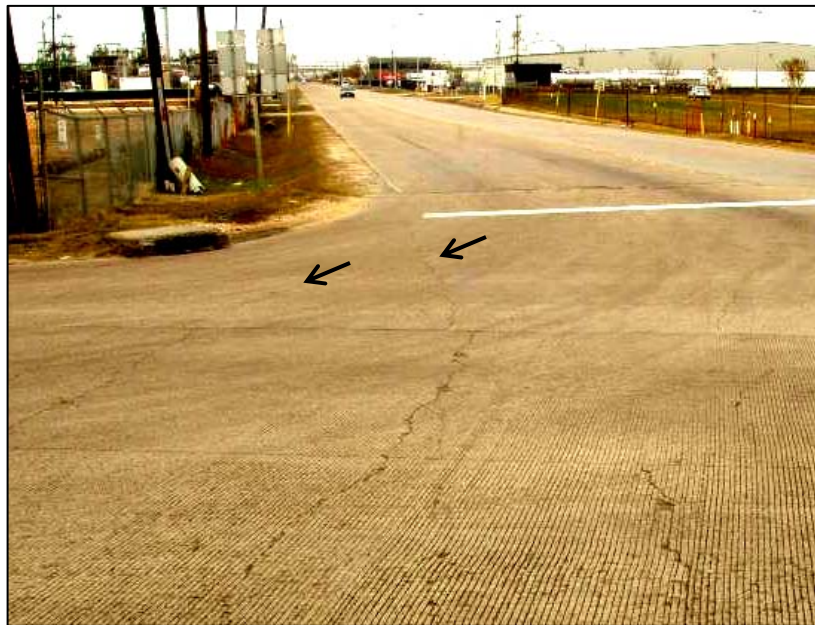
Figure 3-5 Reflection Cracking Associated with Radial Transition.
