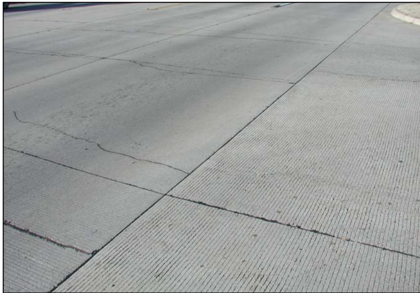
Figure 3-18 Restrained Transverse Cracking.
