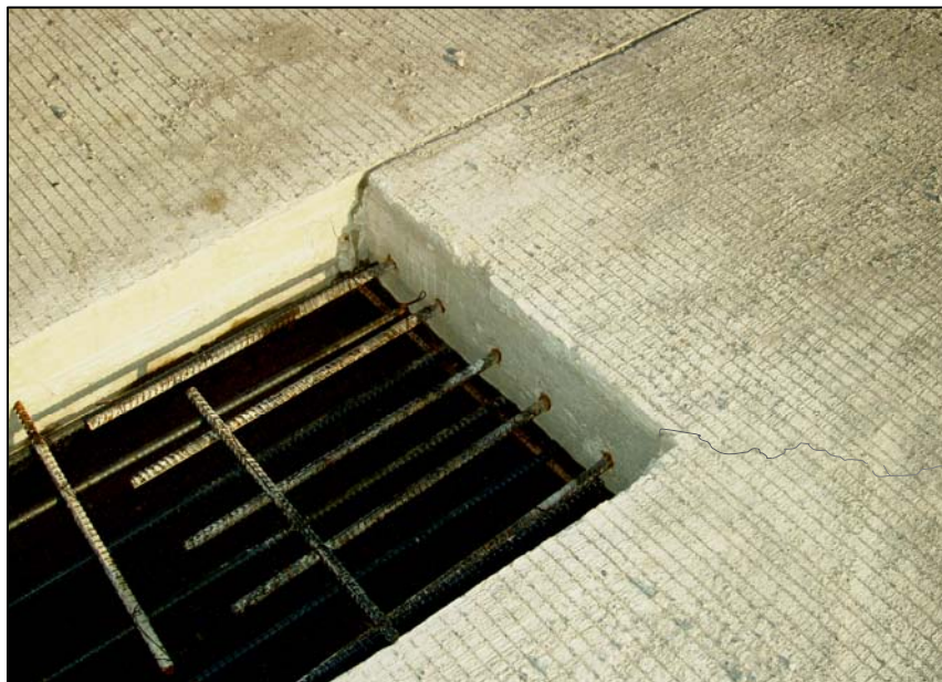
Figure 3-17 Random Diagonal Crack on the Gore Area.
