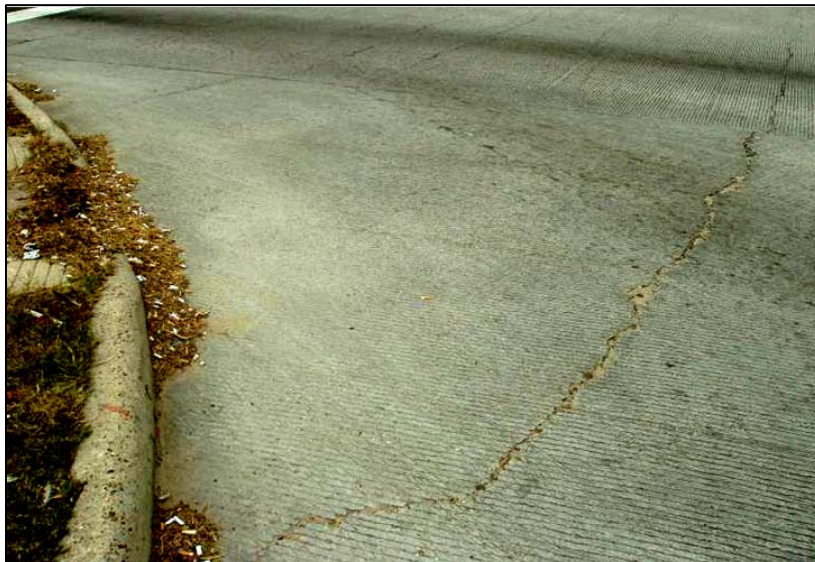
Figure 3-1 Restraint Cracks in the Turning Radius Transition Area.
