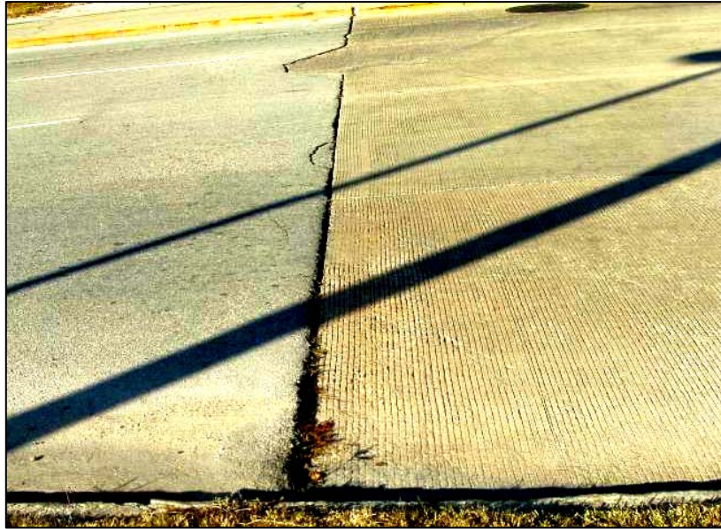
Figure 3-6 Faulted and Spalled AC/PCC Transition Construction Joint.
