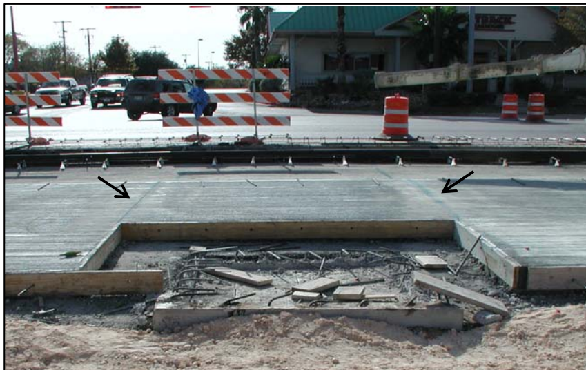
Figure 3-13 Transverse Sawcuts on the Manhole Structure Corner.
