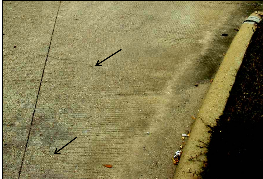
Figure 3-14 Corner Crack in the Turning Radius.
