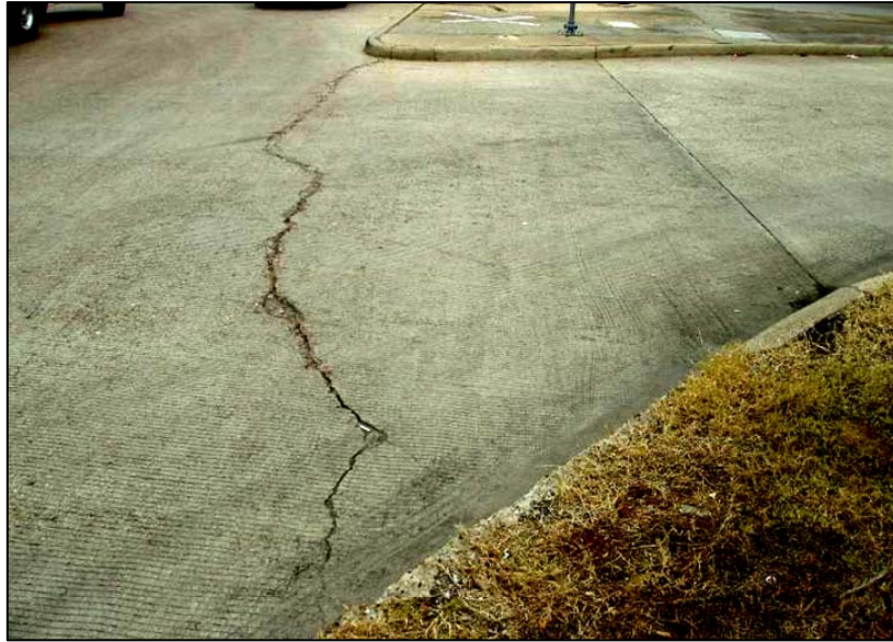
Figure 3-4 Uncontrolled Longitudinal Cracking.
