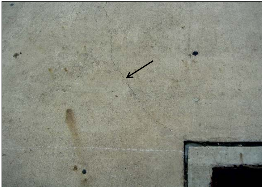
Figure 3-12 Random Diagonal Crack on the Drainage Box Corner.
