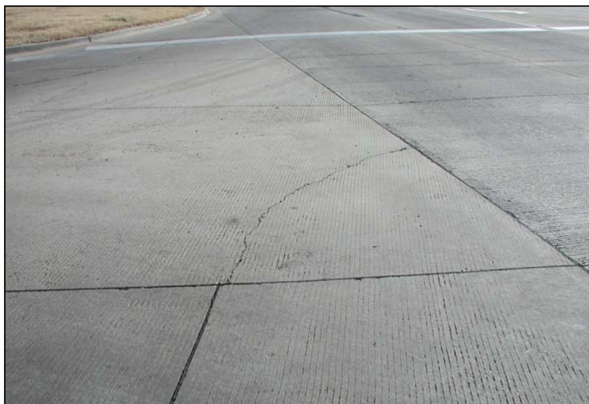
Figure 3-19 Restrained Diagonal Cracking.
