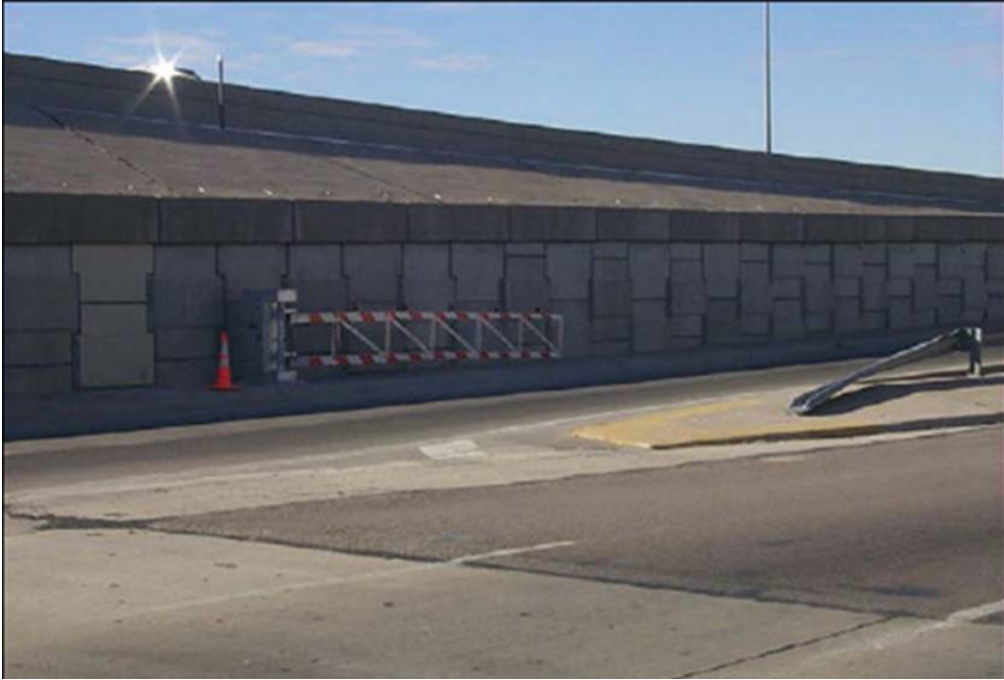
Figure 95. Focus Group Slide 17 Showing Ramp Gate.
