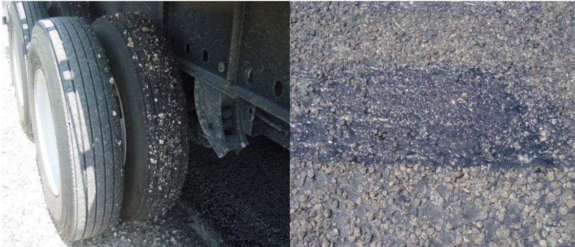
Figure 29. High Level of Damage.
