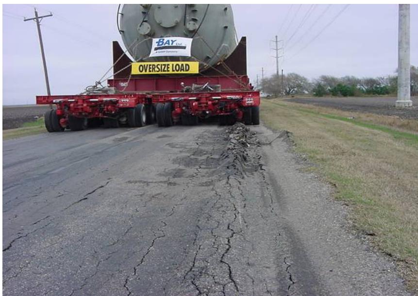
Figure 5. Severe Damage on FM 796.
