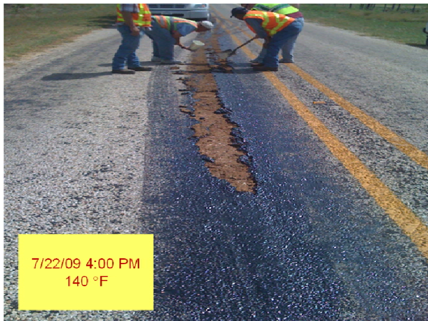
Figure 39. Severe Damage of Surface Treatments.
