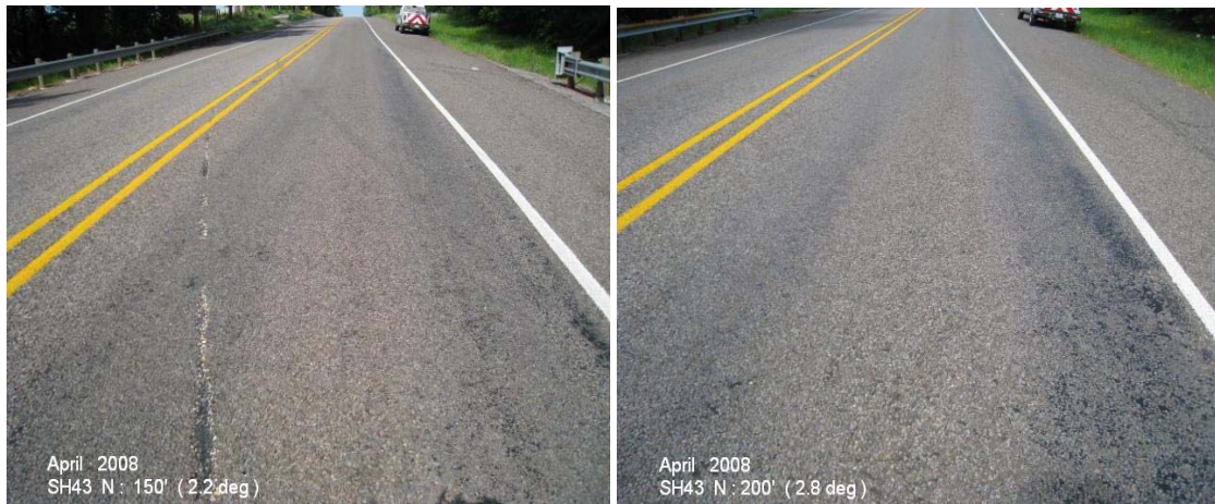
Figure 8. Seal Coat Damage along with Slope.
