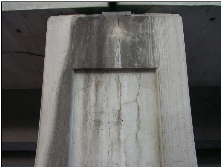
Figure 2. Examples of DEF-Induced Damage in Texas.
