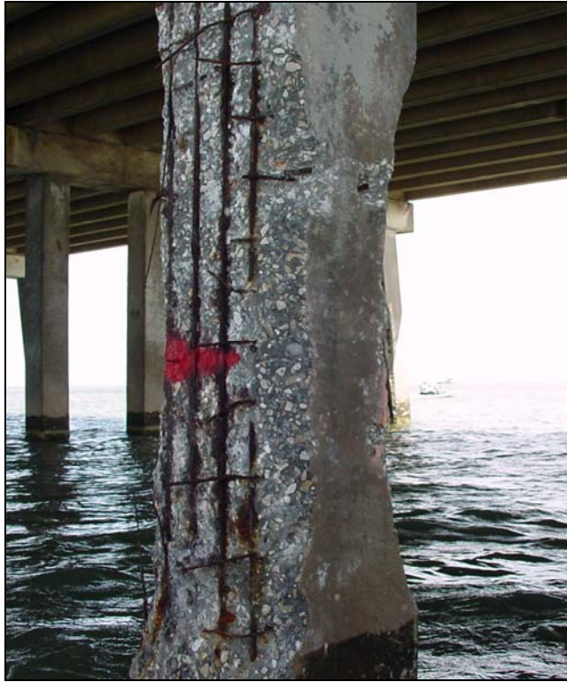
Figure 6. A Close-up View of Corrosion of Reinforced Concrete.
