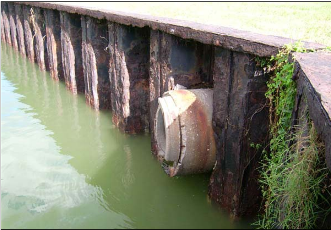
Figure 46. Corrosion of Steel Sheet Piles and Reinforced Concrete Sewer Pipe on Site.
