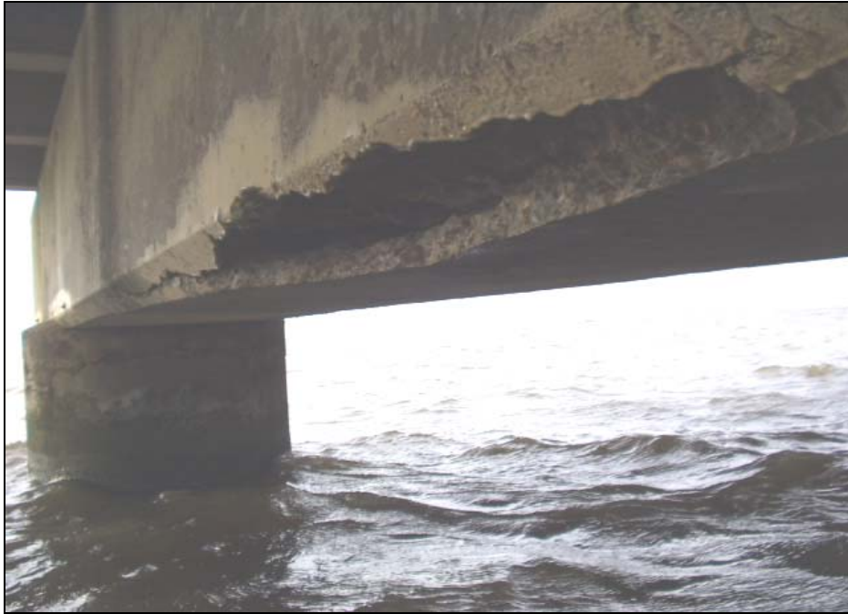
Figure 4. Corrosion of Reinforced Concrete Bent.
