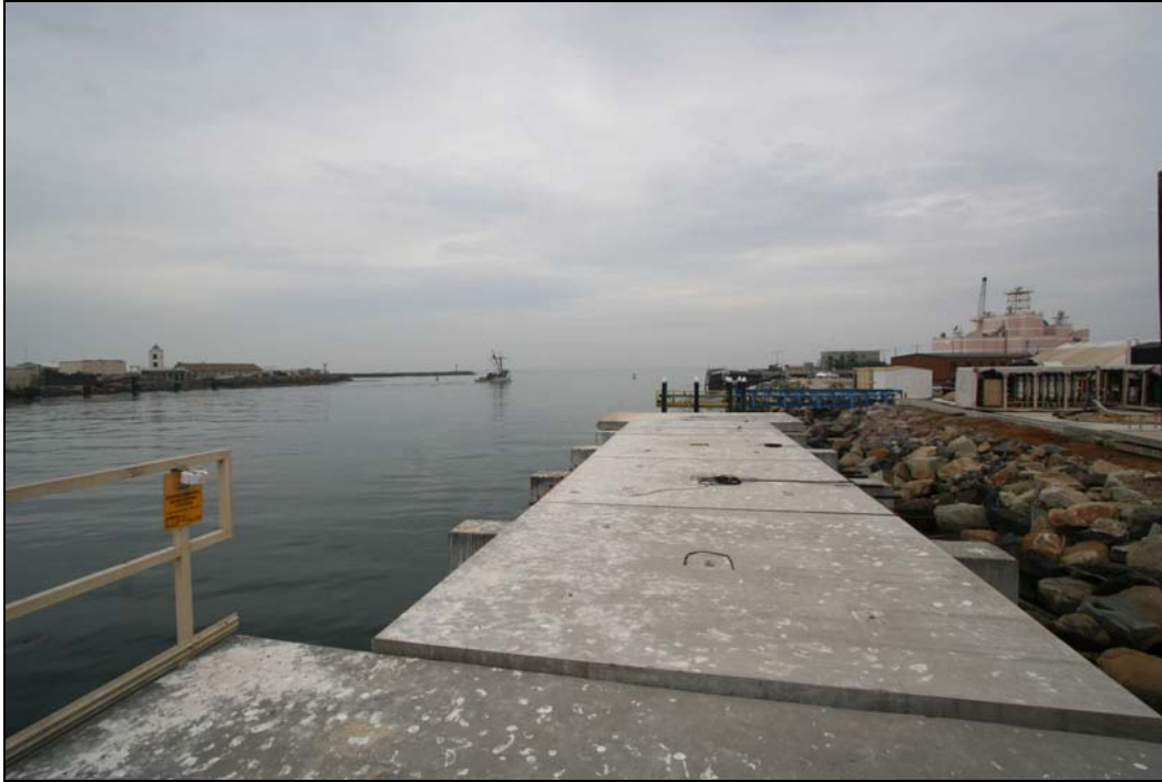
Figure 33. Exposed Pier Slabs.
