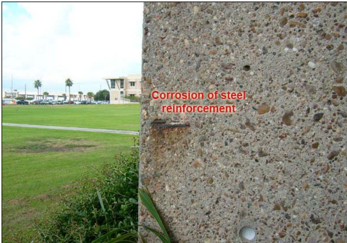
Figure 44. Corrosion of Steel Tie in a Reinforced Concrete Column on Site.
