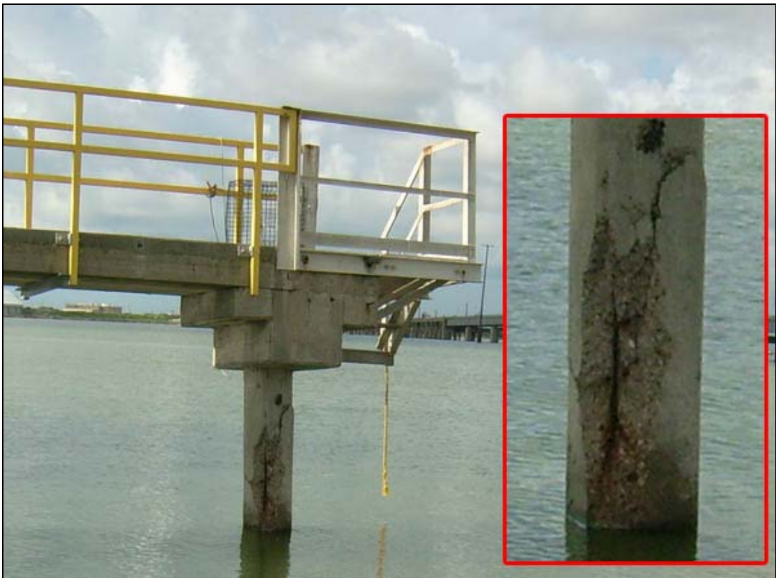
Figure 48. Degradation of a Reinforced Concrete Pile on Site.
