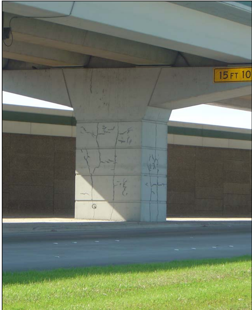
Figure 1. Examples of ASR-Induced Damage.
