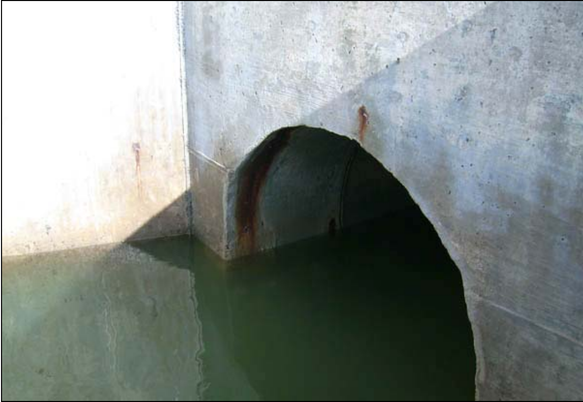
Figure 45. Corrosion of Steel Reinforcement on Site.
