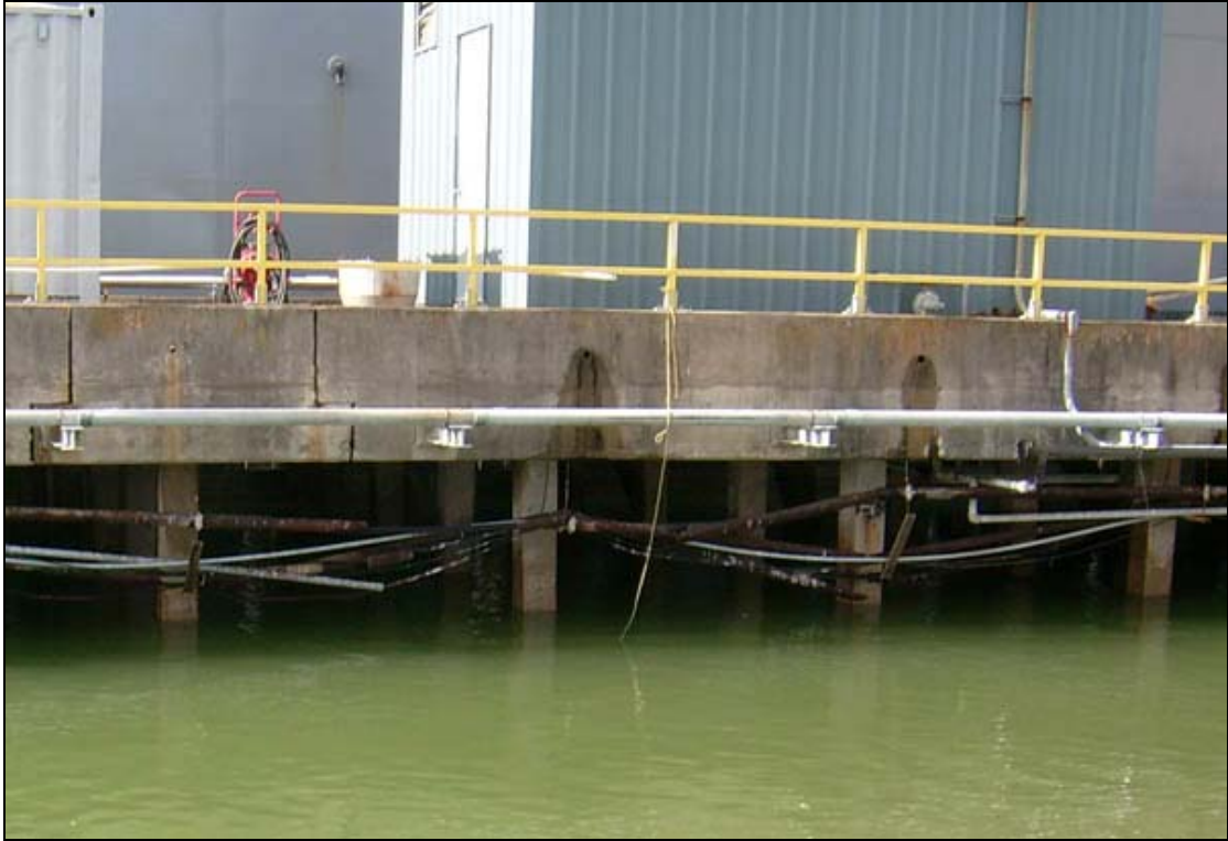
Figure 47. Corrosion of Steel Pipes on Site.
