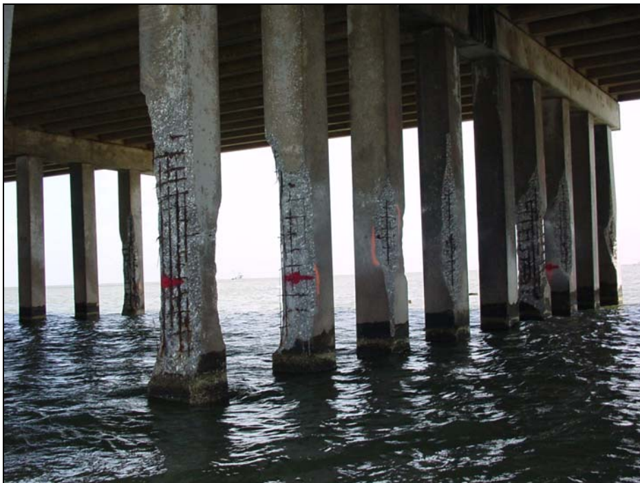
Figure 5. Spalling and Strand Corrosion.
