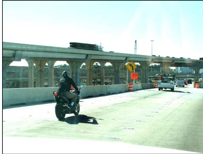
Figure 16. Combination of Permanent and Temporary Warning Signs.
