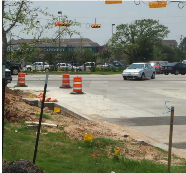
Figure 15. Drop-off near a Sidewalk Edge.
