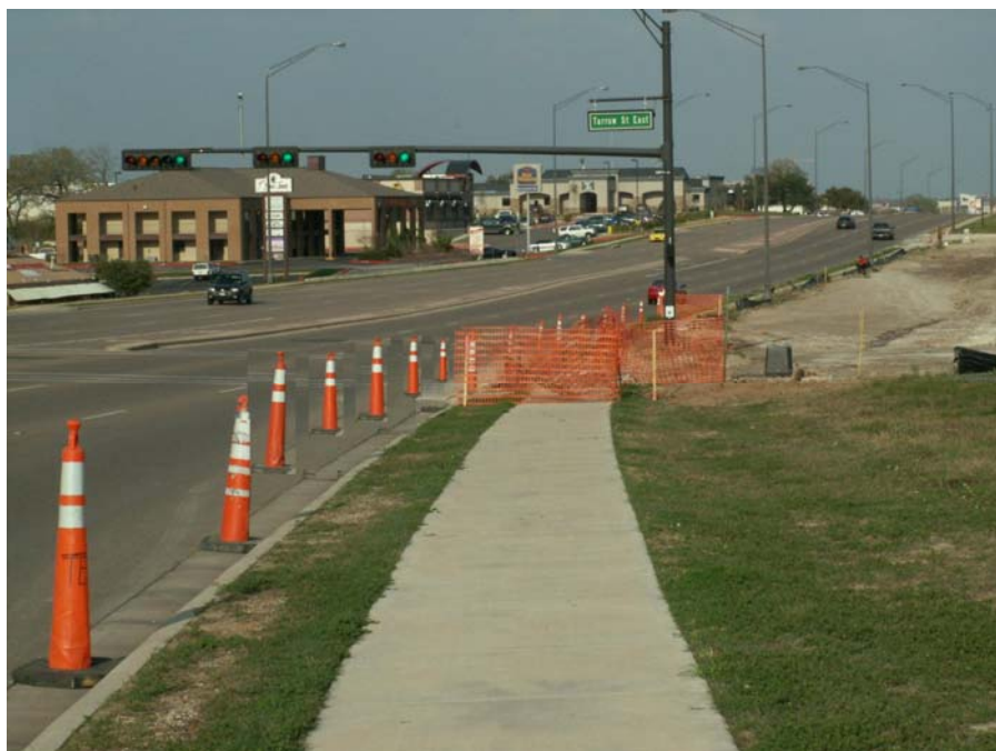
Figure 17. Alternate Path Provided in Roadway.
