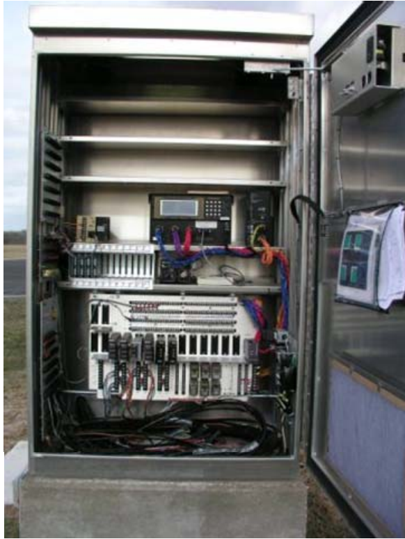
a. Cabinet without AWEGS Equipment
