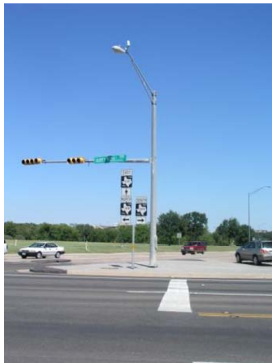
Figure 18. Installation of a Video Detection System for Evaluating Red-Light Runners.
