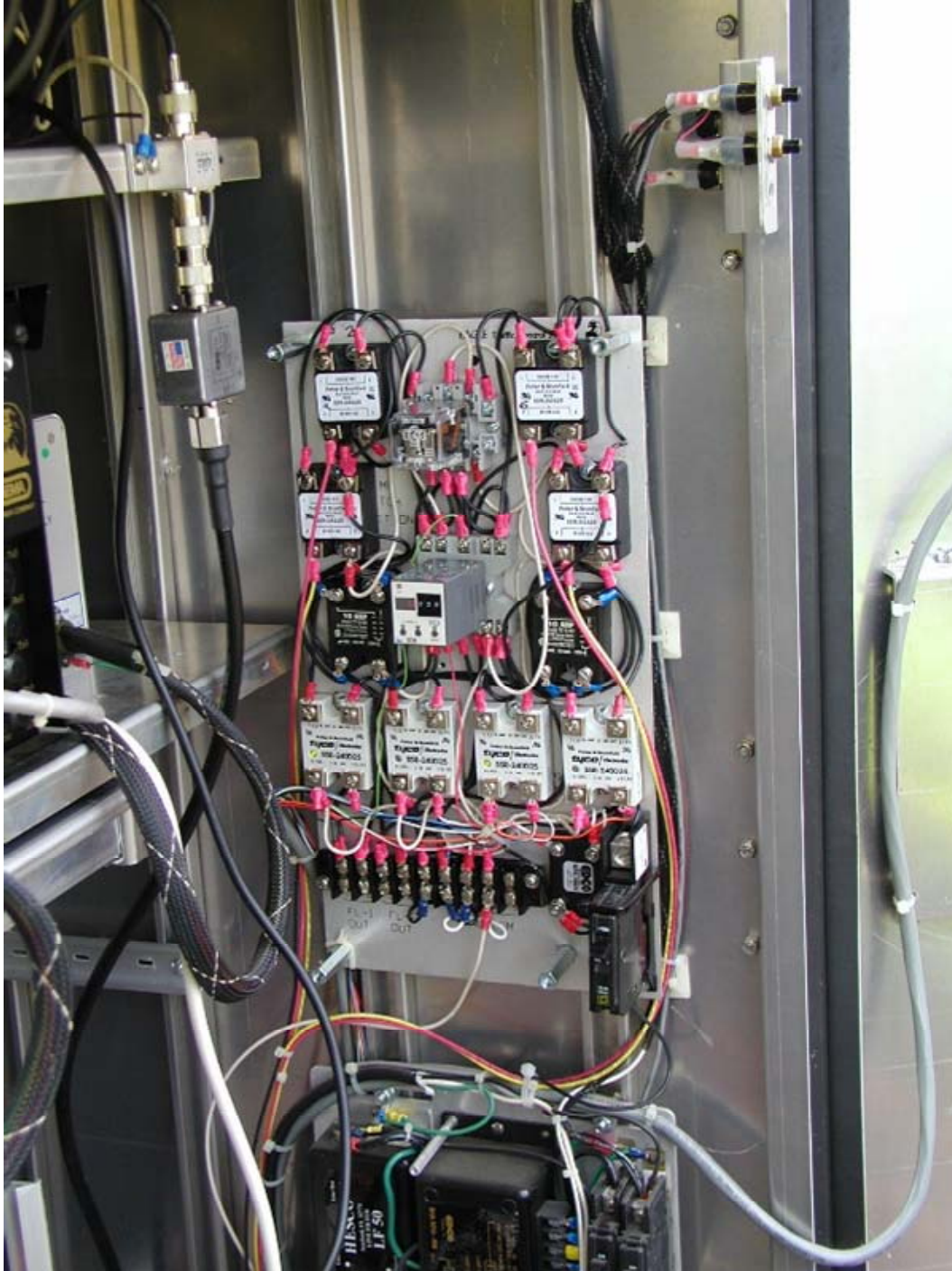
Figure 14. Flasher Panel Installed in a Cabinet.
