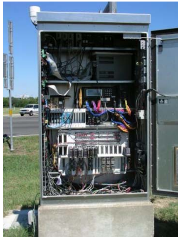
b. Cabinet with AWEGS Equipment
