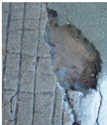
Figure 5.2 Spall Damage at Location 2
