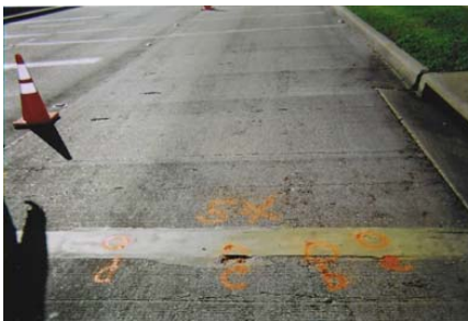
Figure 5.7 Spall Damage at Location 5
