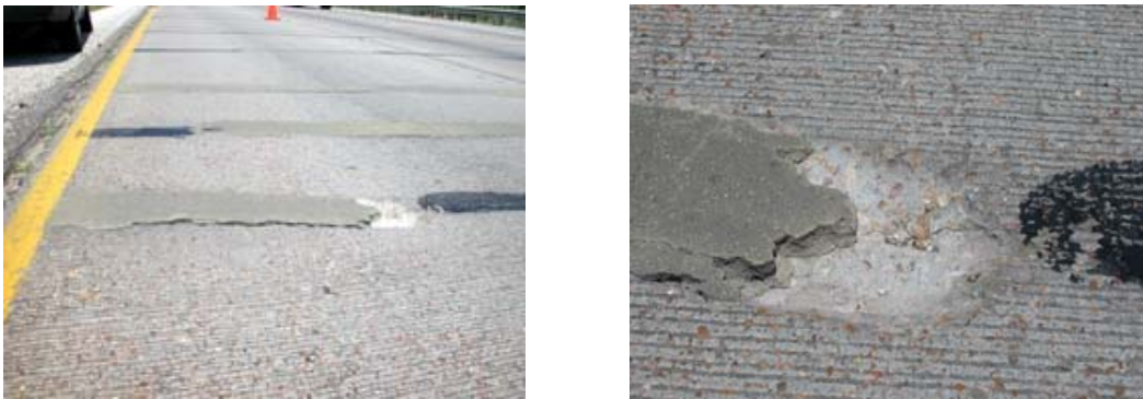
Figure 5.13 De-bonding of Repair Material at Location 11
