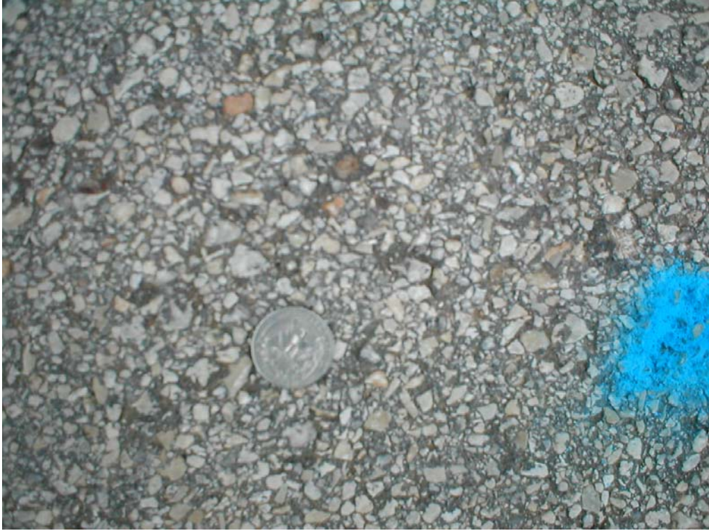
Figure B-17. Carrizo Springs Airport, Untreated Surface Close-up (2006).
