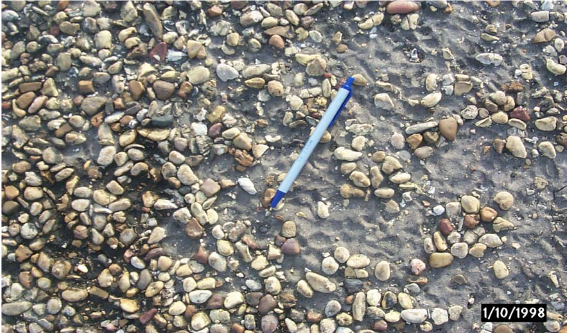
Figure 1-13. Aged Pavement with Raveling.
