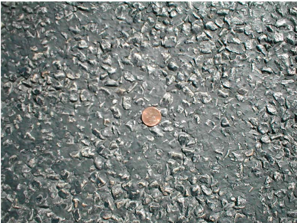
Figure B-26. Fort Worth, FM 4, 2003, Treated COS-50 Close-up (2006).
