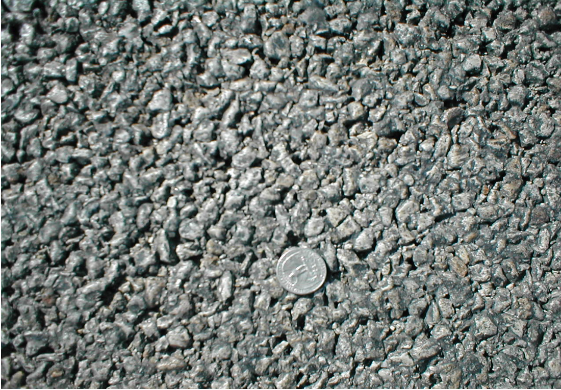
Figure B-7. Abilene, SH 36 R1, Untreated Surface Close-up (2006).
