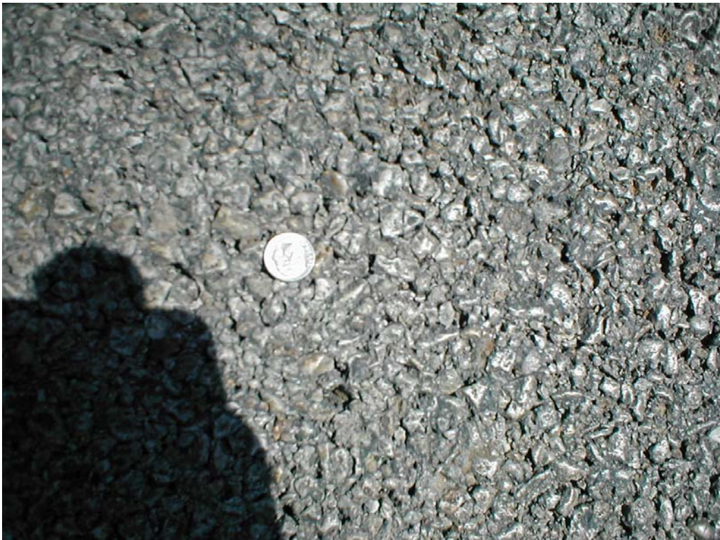
Figure B-6. Abilene, SH 36 L2 Untreated Surface Close-up (2006).
