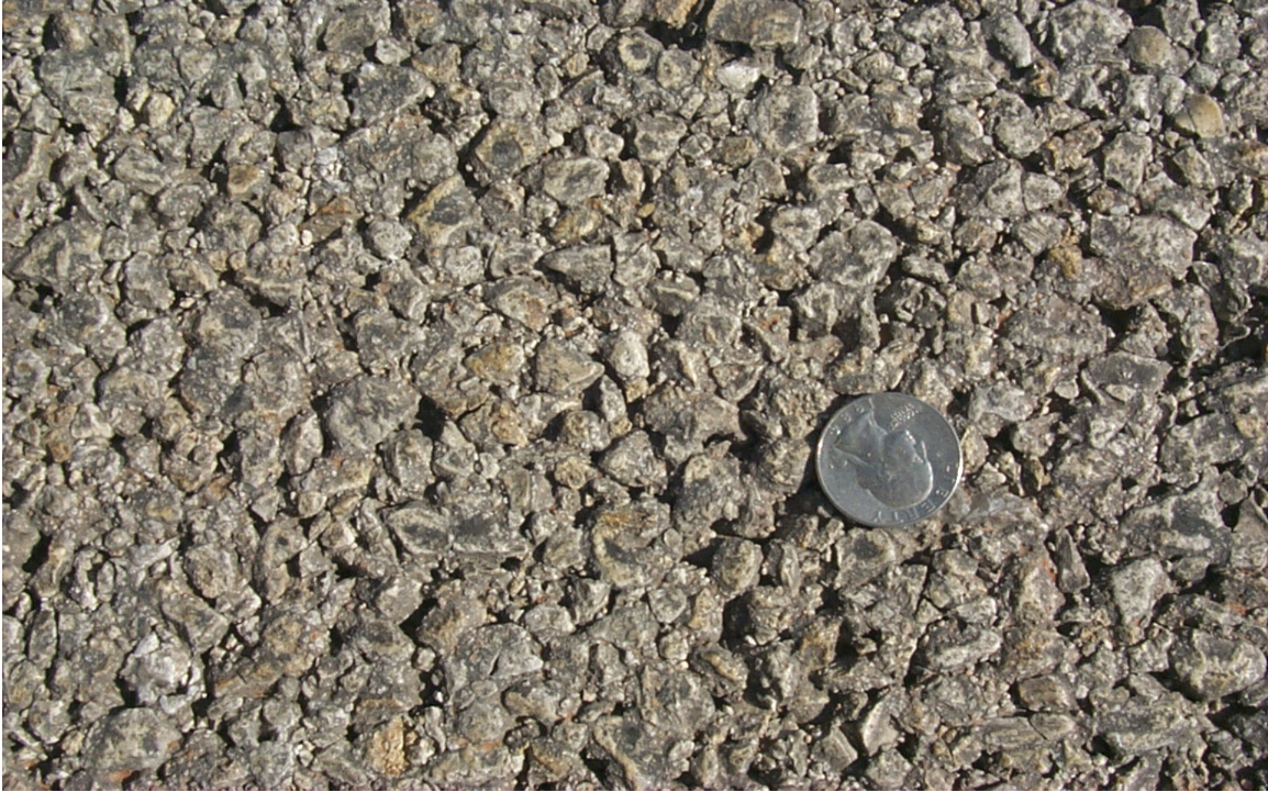
Figure B-3. Abilene, SH 36 L2, Untreated Surface, Close-up (2004).
