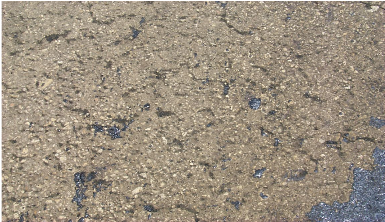
Figure 1-6. Unsealed, Aged Pavement.
