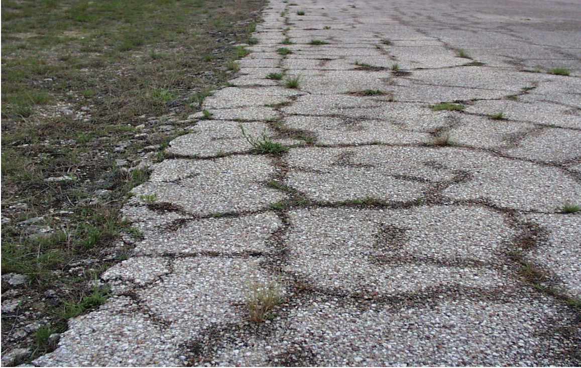
Figure 1-7. Block Cracked Pavement.
