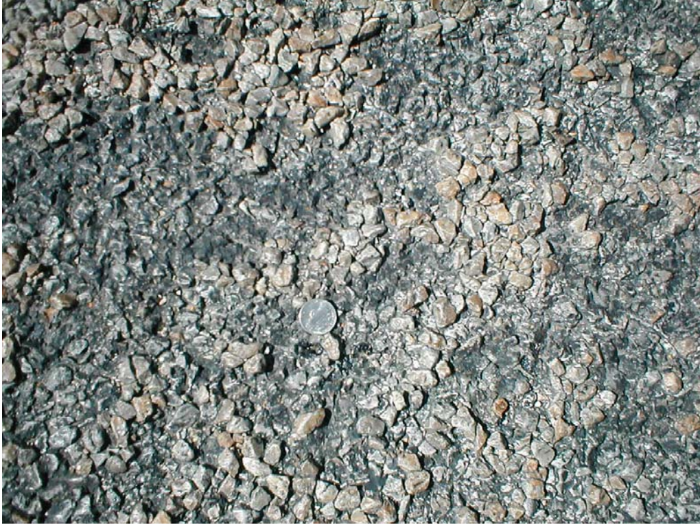
Figure B-21. Fort Worth, FM 4, 2000, Untreated Surface Close-up (2006).
