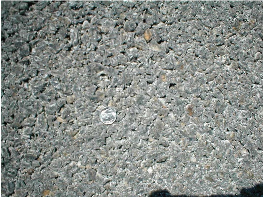
Figure B-8. Abilene, SH 36 R2, Untreated Surface Close-up (2006).
