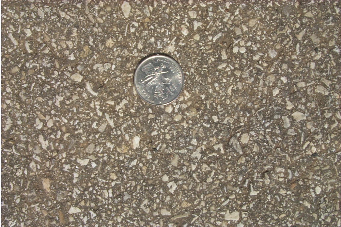
Figure B-15. Carrizo Springs Airport, Untreated Surface Close-up (2004).
