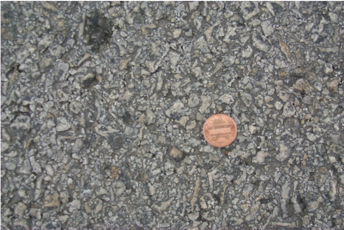
Figure B-4. Abilene, SH 36 R1, Untreated Surface, Close-up (2004).
