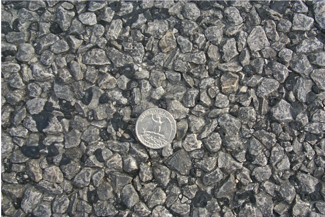
Figure B-23. Fort Worth, FM 4, 2003, Untreated Surface Close-up (2005).
