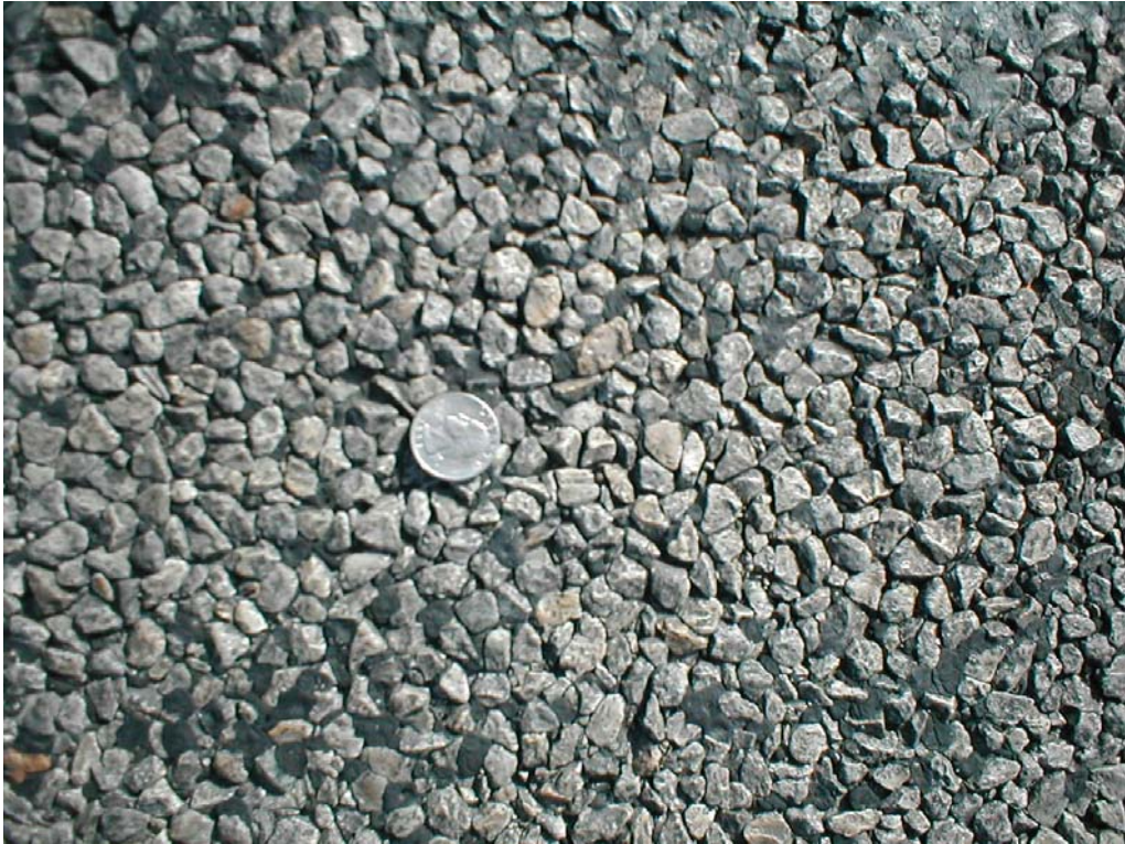
Figure B-25. Fort Worth, FM 4, 2003, Untreated Surface Close-up (2006).
