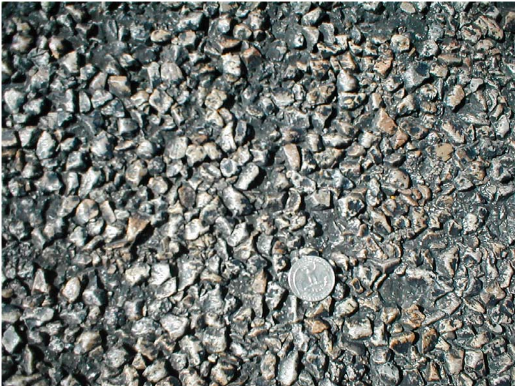
Figure B-22. Fort Worth, FM 4, 2000, Treated COS-50 Close-up (2006).
