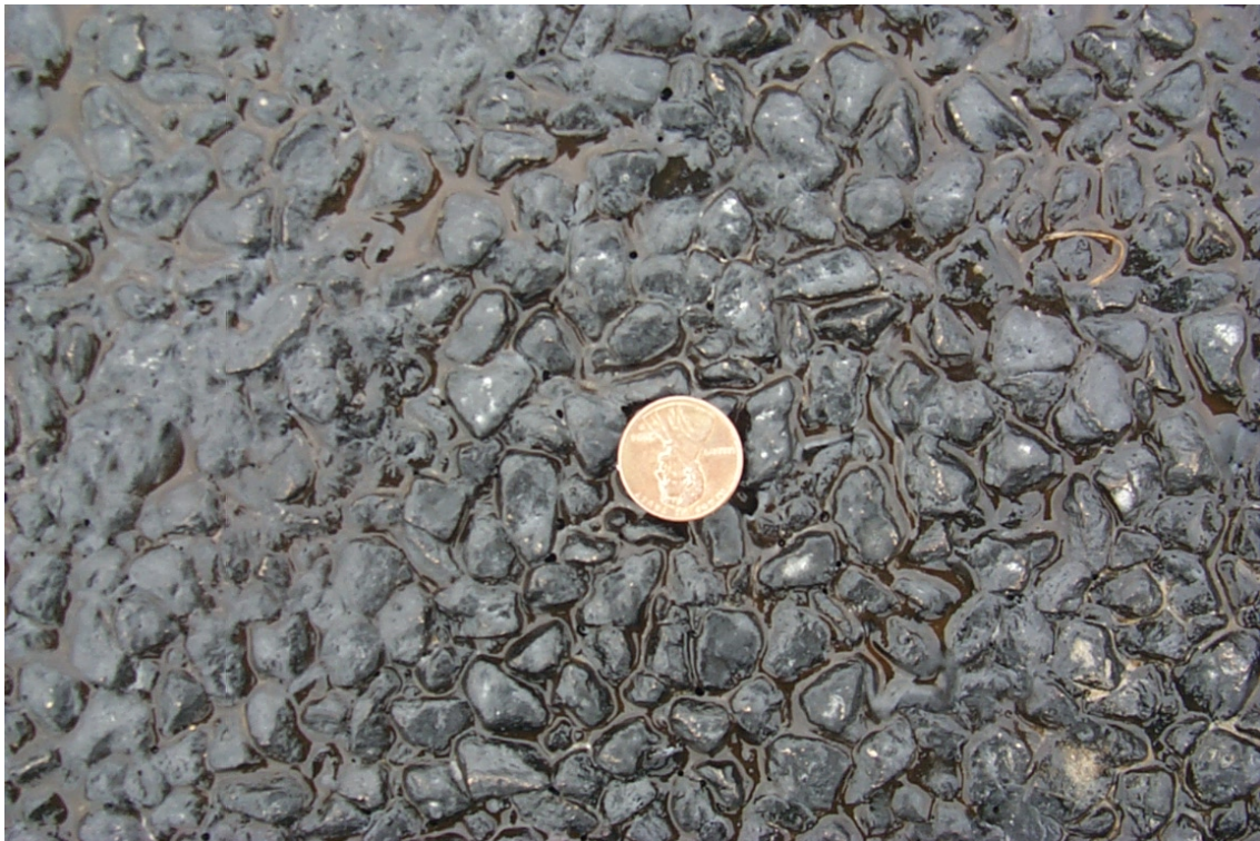
Figure B-20. Fort Worth, FM 4, 2000, Treated COS-50 Close-up (2005).
