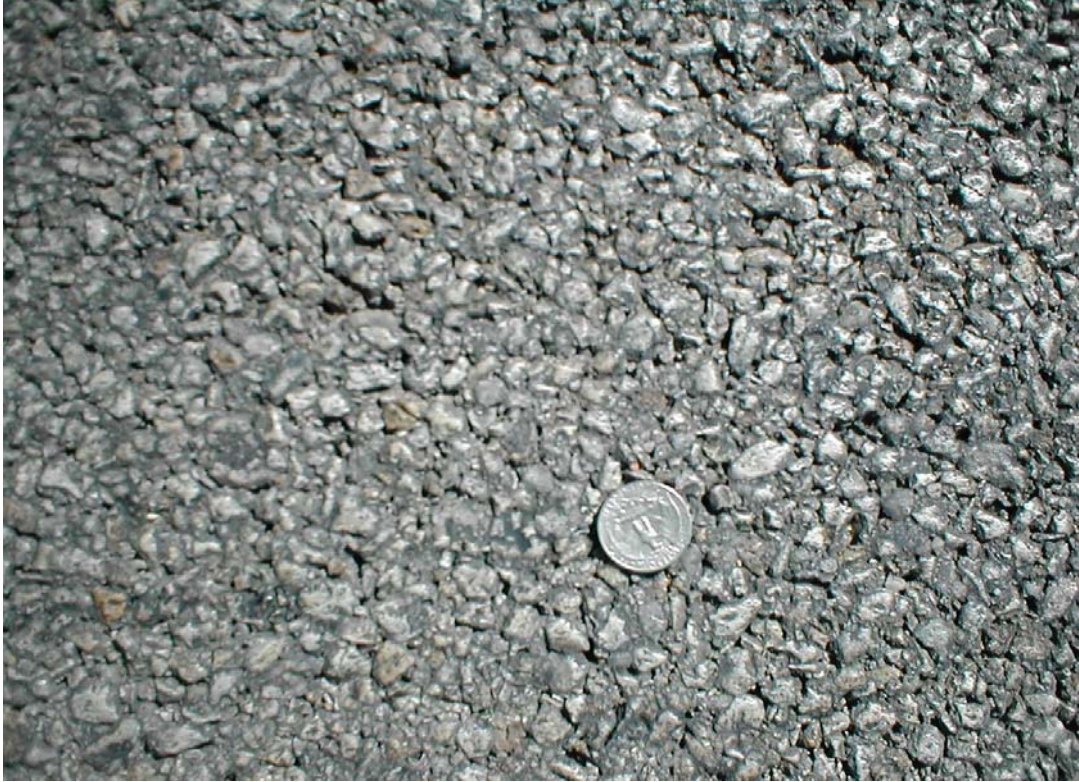
Figure B-5. Abilene, SH 36 L1, Untreated Surface Close-up (2006).
