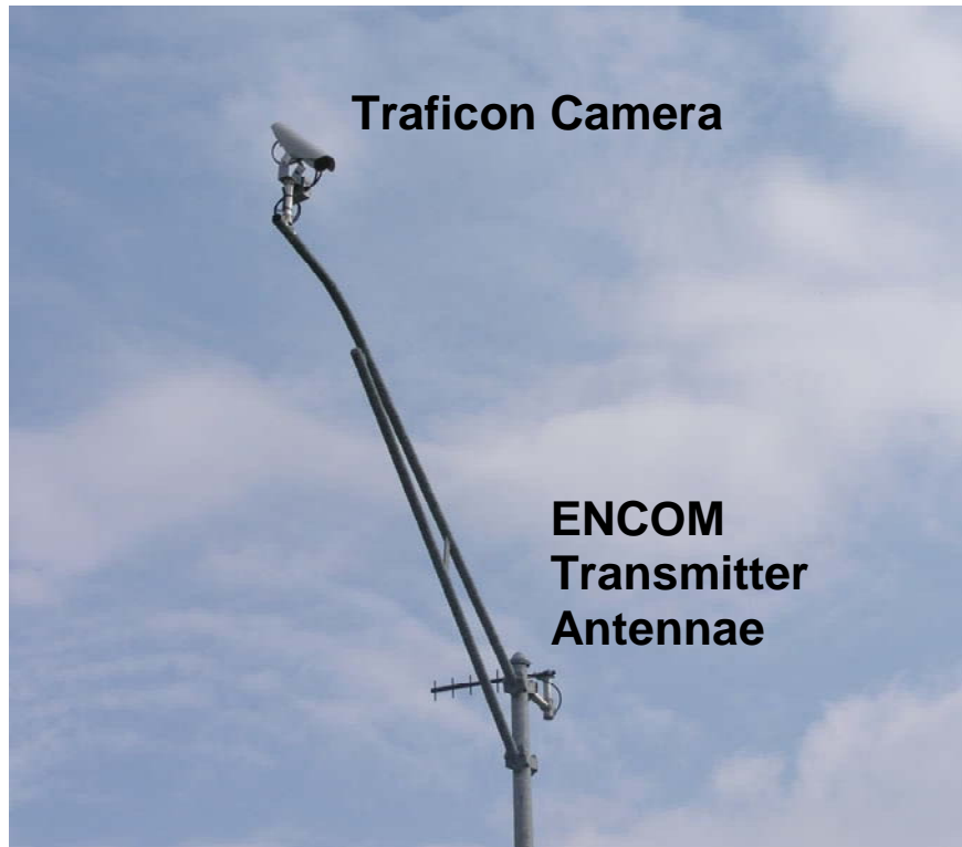
Figure 8. Traficon Camera Installation.
