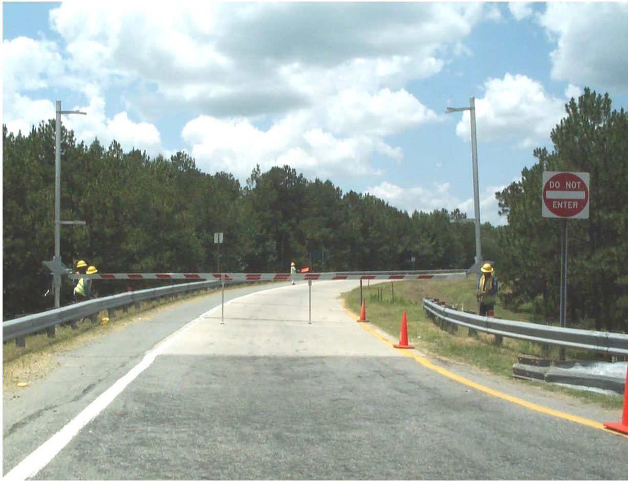
Figure 3. Drop Gate Barricade at Entrance Ramp in Georgia (10).
