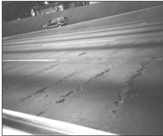
(a) Spalling damage
