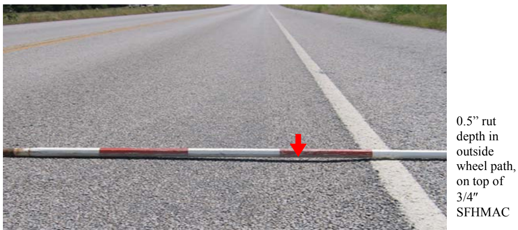
Figure 4-1. Surface Rutting on Top of \frac{3}{4} " SFHMAC Prior to \frac{1}{2} " HDSMA.
