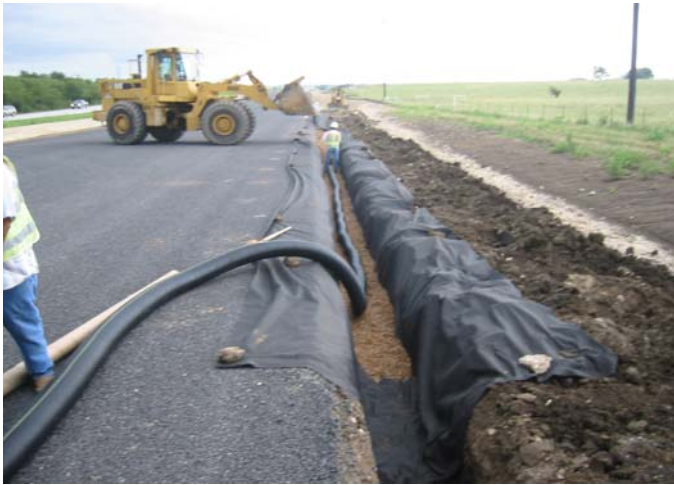
Figure 27. Installing Edge Drains in SH 114 to Drain Water Trapped within the SF Layers.
