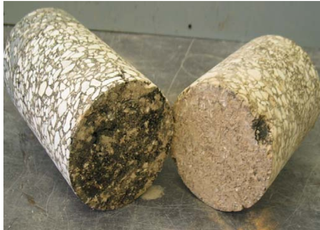
Figure 19. Debonded Core from the Zumwalt 1 Job in Laredo.
