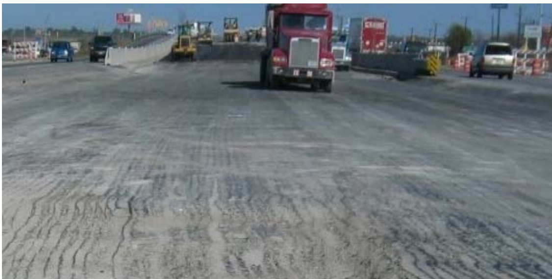
Figure 20. Inadequate Tack Coat on a Perpetual Pavement.
