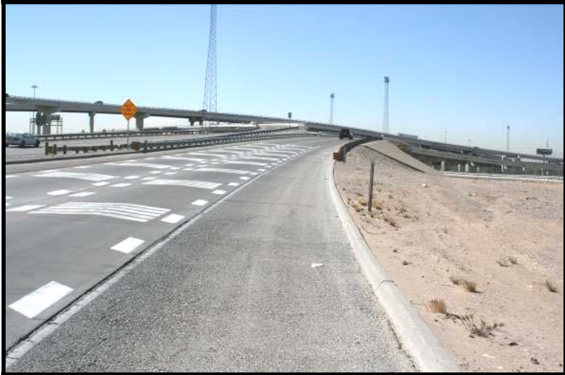
Figure 19. Chevron Markings Ending Near the Beginning of the Connector Curve.
