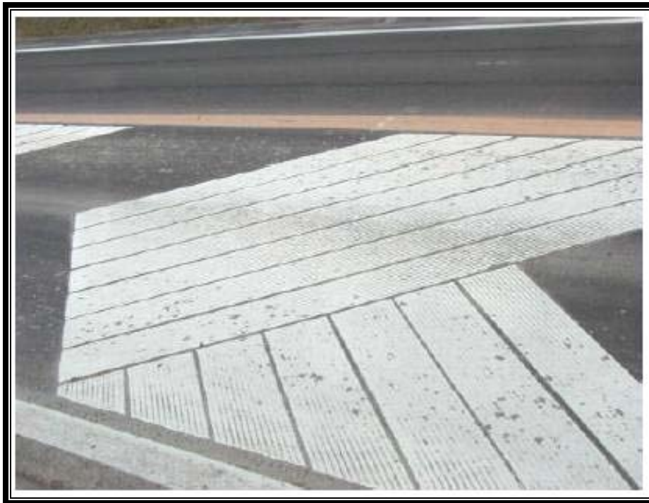
Figure 6. Closer View of Anti-skid Chevron Markings (30).
