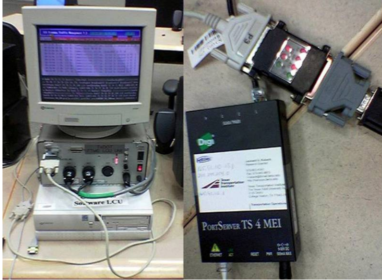
Figure 22. TTI Office LAN, SCU, and Digi Terminal Server.
