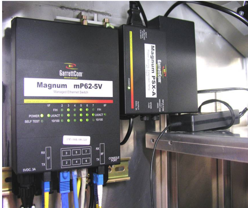
Figure 14. GarrettCom mP62-5V Managed Switch.
