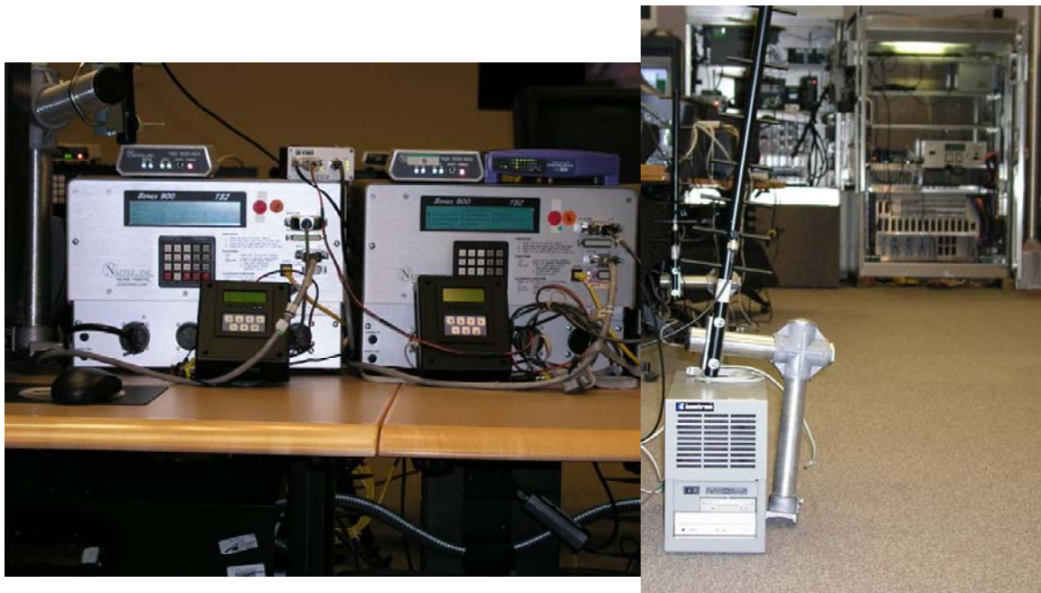
Figure 15. TransLink Installed Master and Slave Subsystems.
