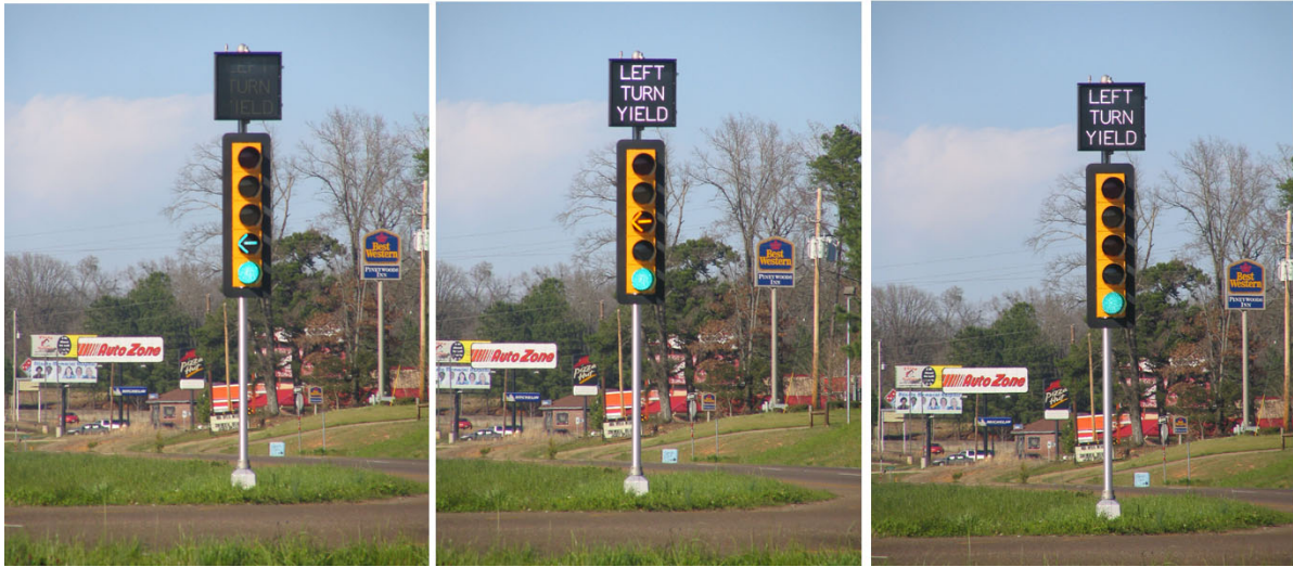
a. Protected Phase EMS not illuminated
