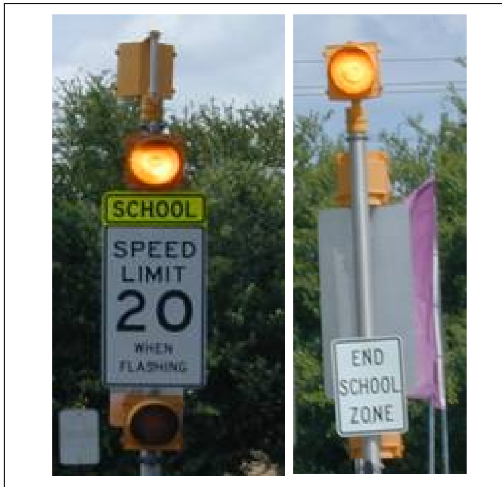
Figure 3-1. Rear-Facing Beacon Installation.
