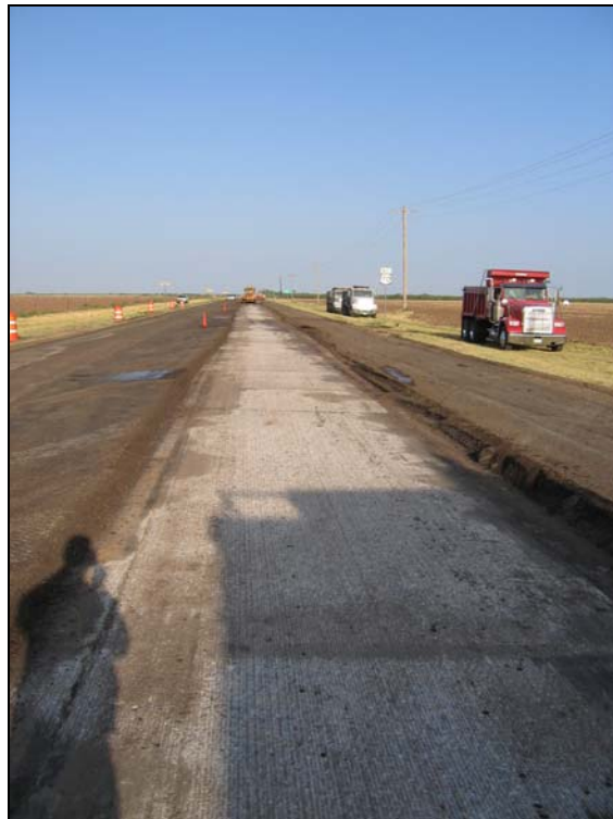
Figure 6.4. Existing Concrete Slabs on US 70 in Foard County.
