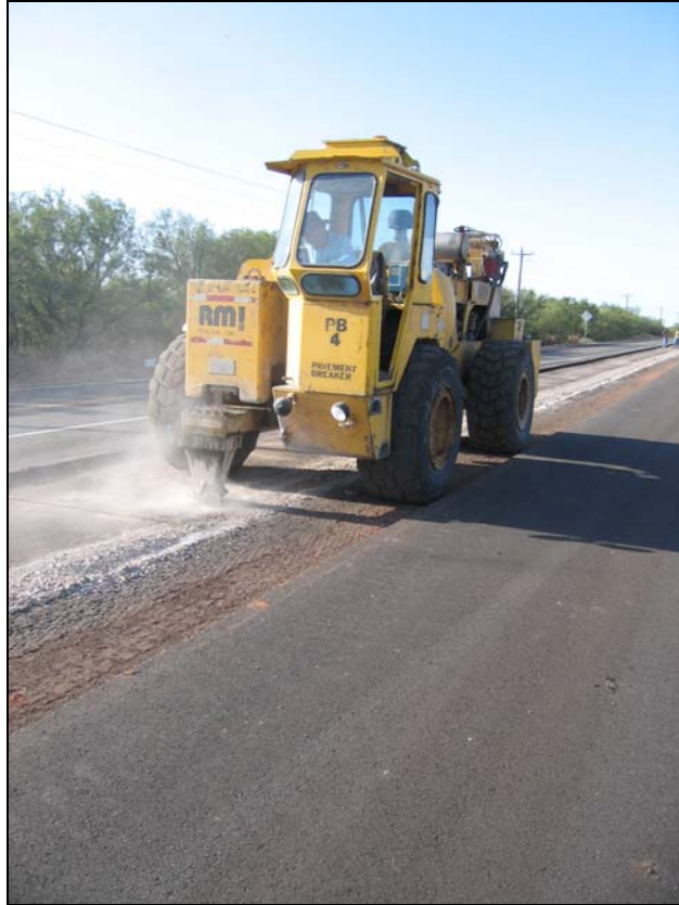
Figure 7.7. Resonant Breaker on US 83 from King/Cottle County Line.
