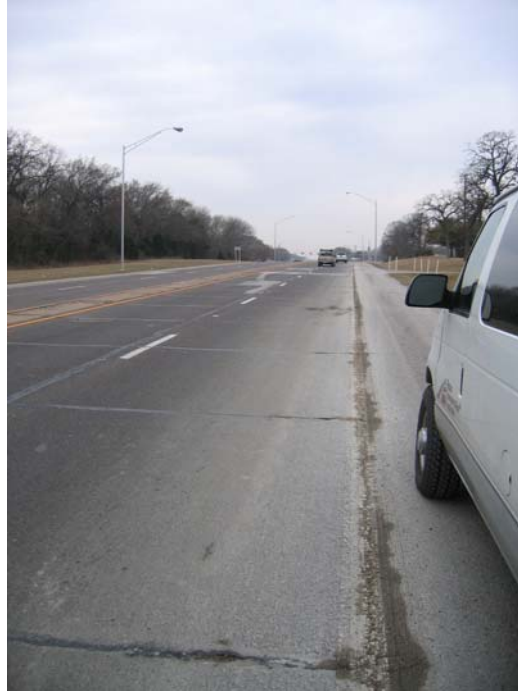
Figure 4.1. Representative Pavement Condition on Loop 12.
