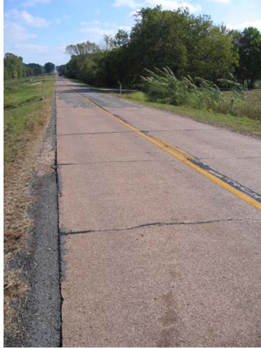
Figure 1.1. Cracked Slabs on FM 912.
