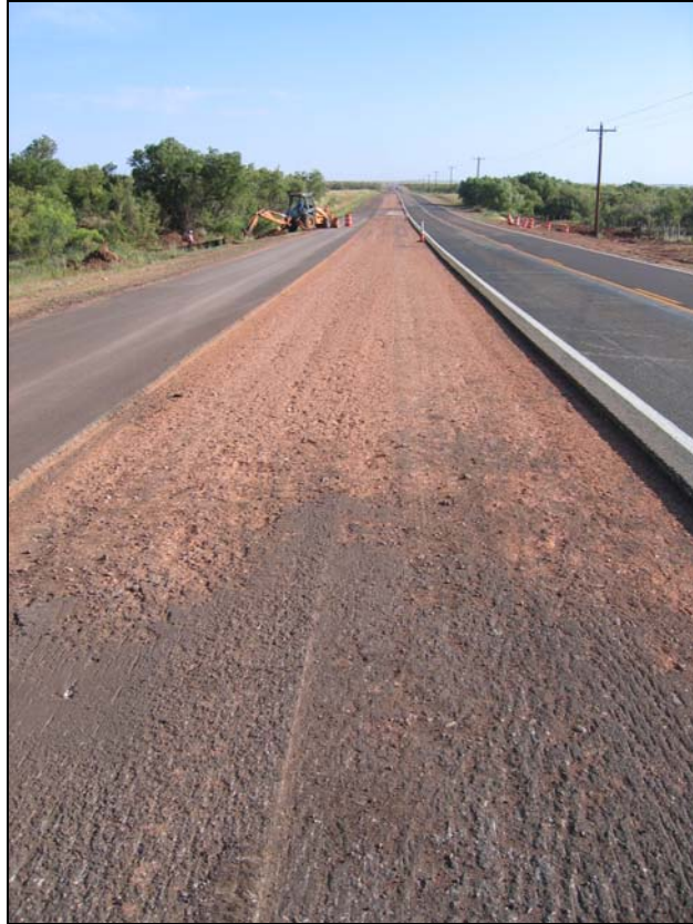
Figure 7.12. Location of Prior Concrete Removal on US 83 from King / Cottle County Line.
