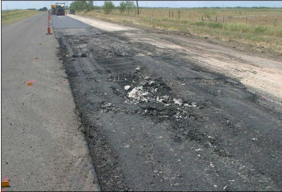
Figure 6.7. Failure on US 70 Encountered during Paving.
