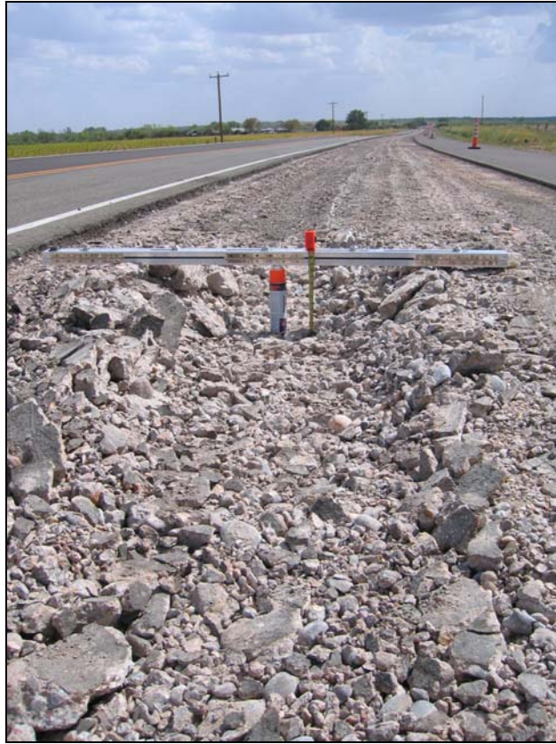
Figure 7.11. Rutting in Rubblized Layer from Resonant Breaker.
