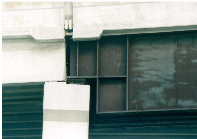
Figure 1-2. Example of Welded Dapped Girder Detail (Sam Houston Tollway and Interstate 10 Interchange, Houston, TX).
