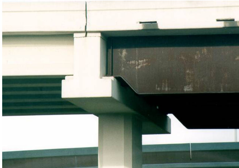
Figure 1-1. Example of Bridge Bent Cap Supporting Both a Steel Girder and Prestressed Concrete Beam (U.S. Highway 59 and Sam Houston Tollway Interchange, Houston, TX).
