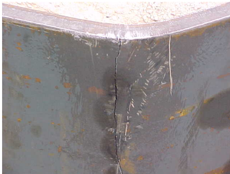
Figure 1-5. View of Cracked Flange Plate As a Result of Bending Operation.
