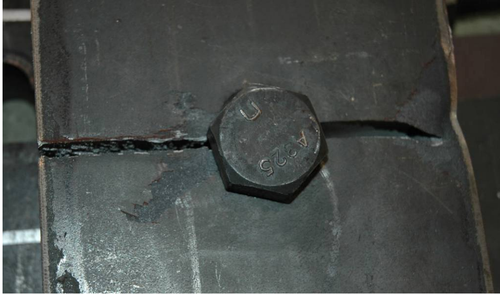
Figure 5-9. Typical Crack Orientation for Thick Plates ( \geq 1.0 Inches) with a Gusset Plate (Specimen E-3).
