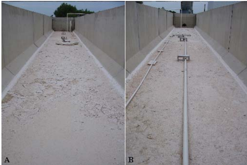
Figure 2.6. View of Sedimentation Tank After Outlet Relocation. A. From Upstream. B. From Downstream.
