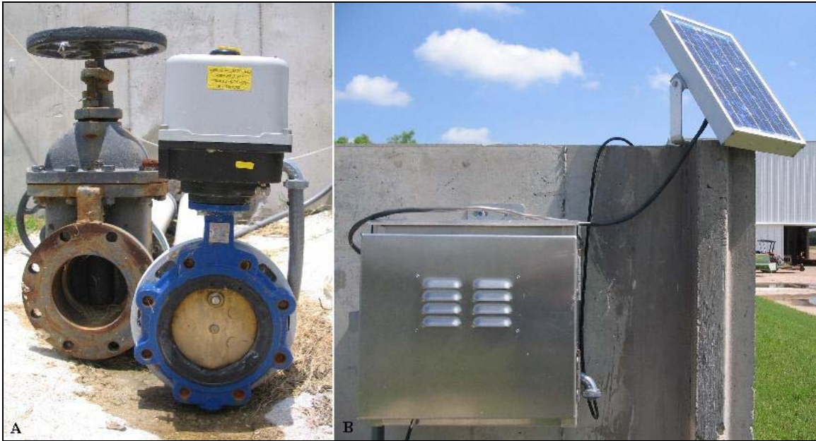
Figure 2.5. A. Gate Valve and Butterfly Valve. B. Actuator Box and Solar Panel.
