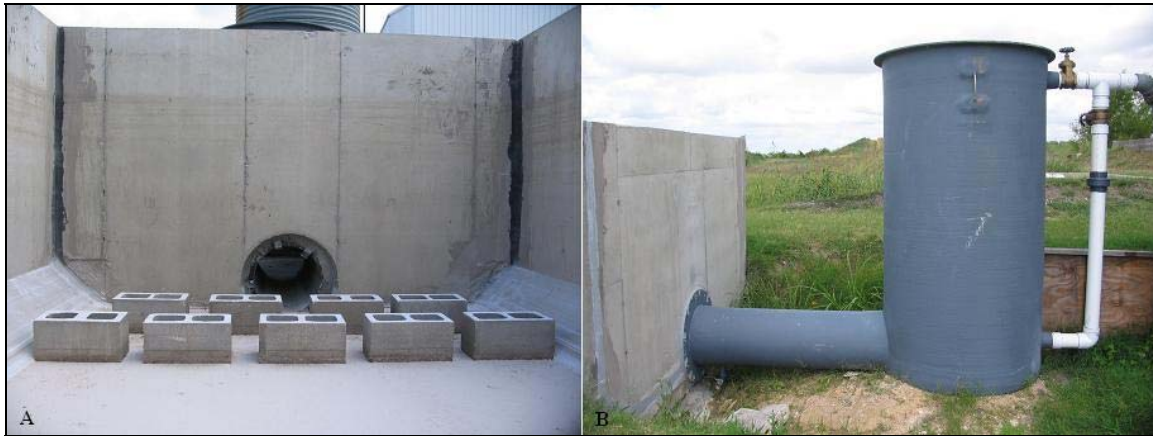
Figure 4.2. A. Energy Dissipation at Inlet. B. Mixing Tank.
