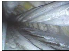
Voids inside PT ducts
