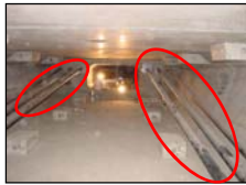
PT ducts inside a typical segmental box girder
