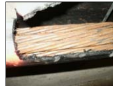
Corroded strands inside PT ducts with voids
