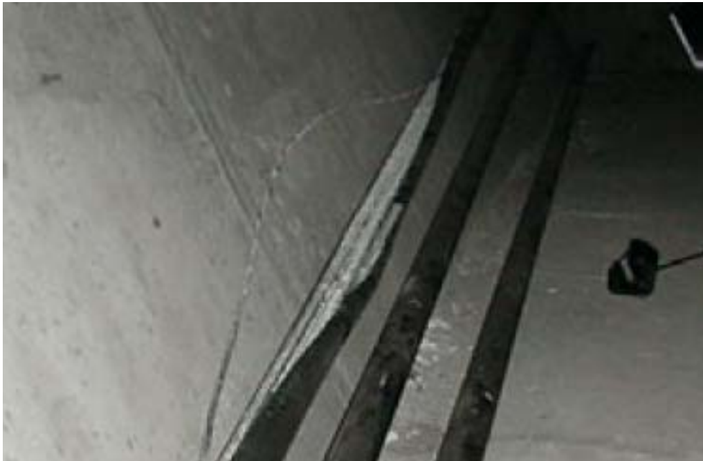
Figure A. Broken strands and broken ducts.
