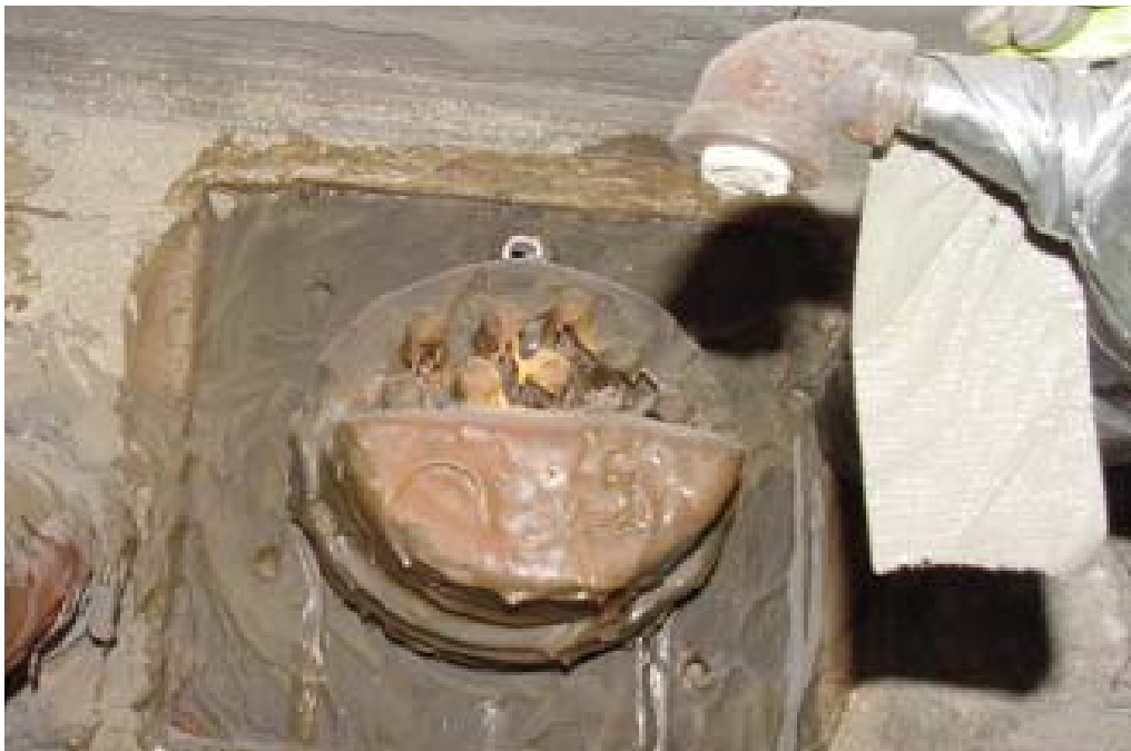
Figure L. Opened grout port, broken anchorage cap, and exposed anchorage zone.
