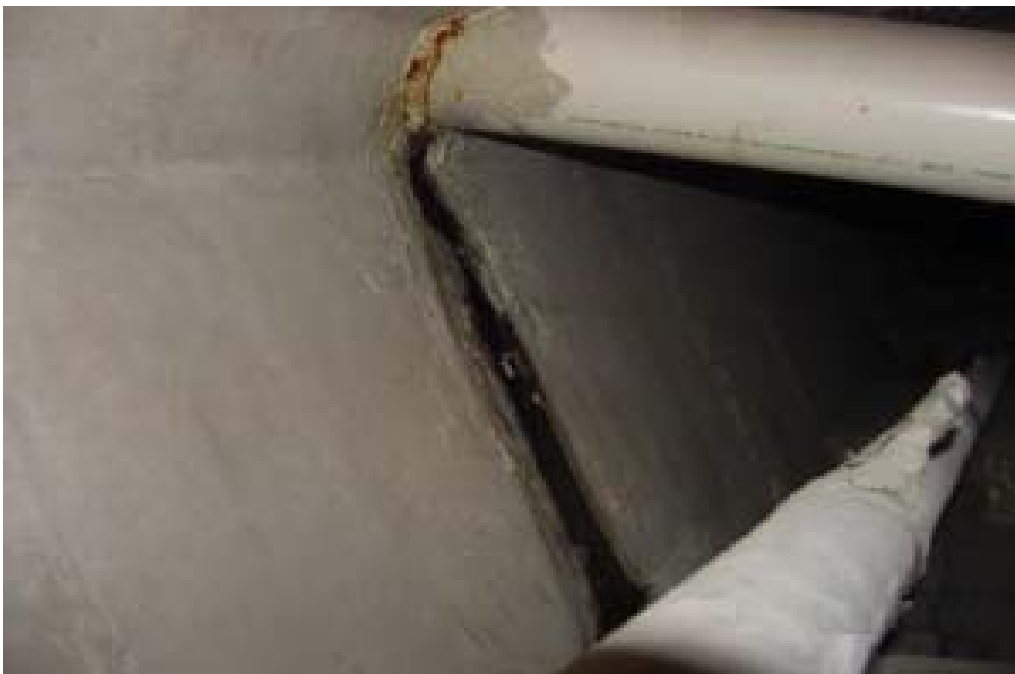
Figure P. Sign of past moisture infiltration in the concrete girder, broken drainage pipe.
