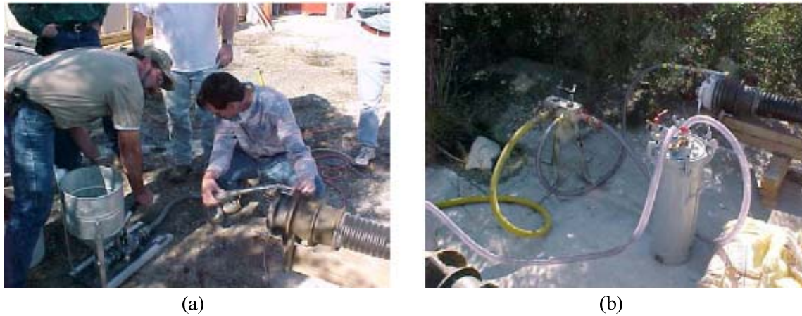
Figure 2-6. Grouting tests conducted by FDOT: (a) Pressure grouting and (b) Vacuum grouting methods (FDOT 2001).
