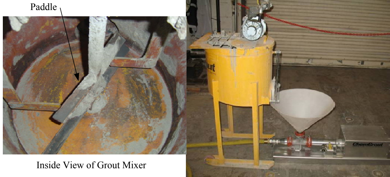
Figure 5-1. Grout Mixer for Initial Grouts and Grout Pump.
