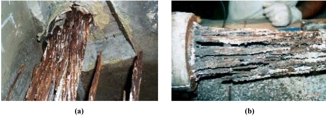
Figure 2-6. Severely Corroded Strands at Anchorage Zones of PT Columns in the Bob Graham Sunshine Skyway Bridge, Tampa Bay, Florida (FDOT 2001b).
