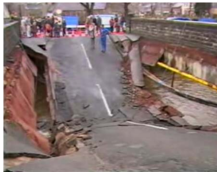
Figure 2-1. Collapsed Ynys-y-Gwas Bridge ( YouTube 2009 ).
