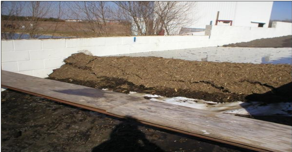
Figure 4.4. Displacement Causing Stresses Leading to Failure of the YWC Berm.
