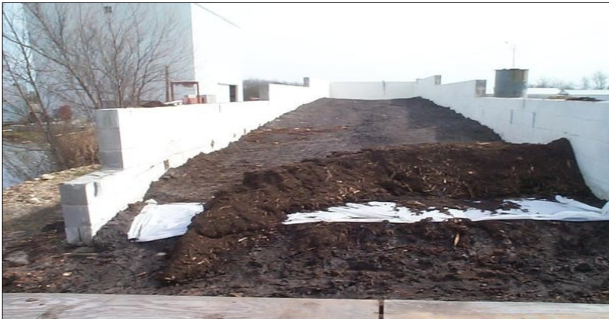
Figure 4.2. Failure of the DMC Berm on Clay Due to Displacement (Round 2-1).
