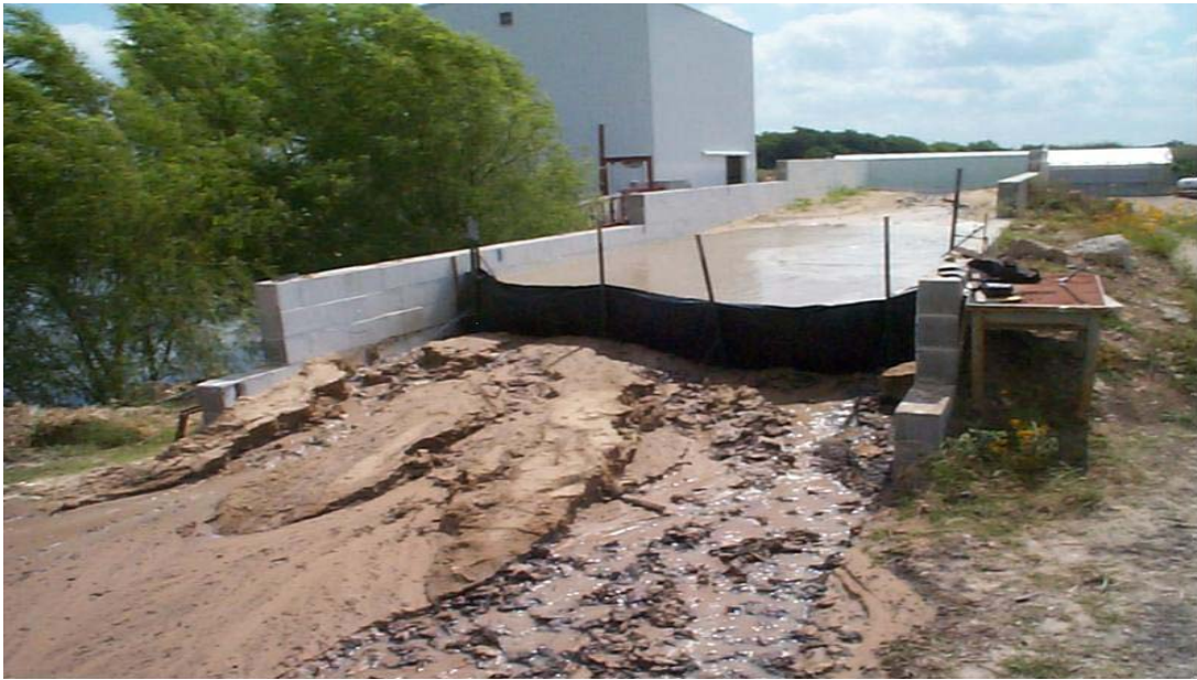
Figure 4.14. Scouring Downstream of the Silt Fence.
