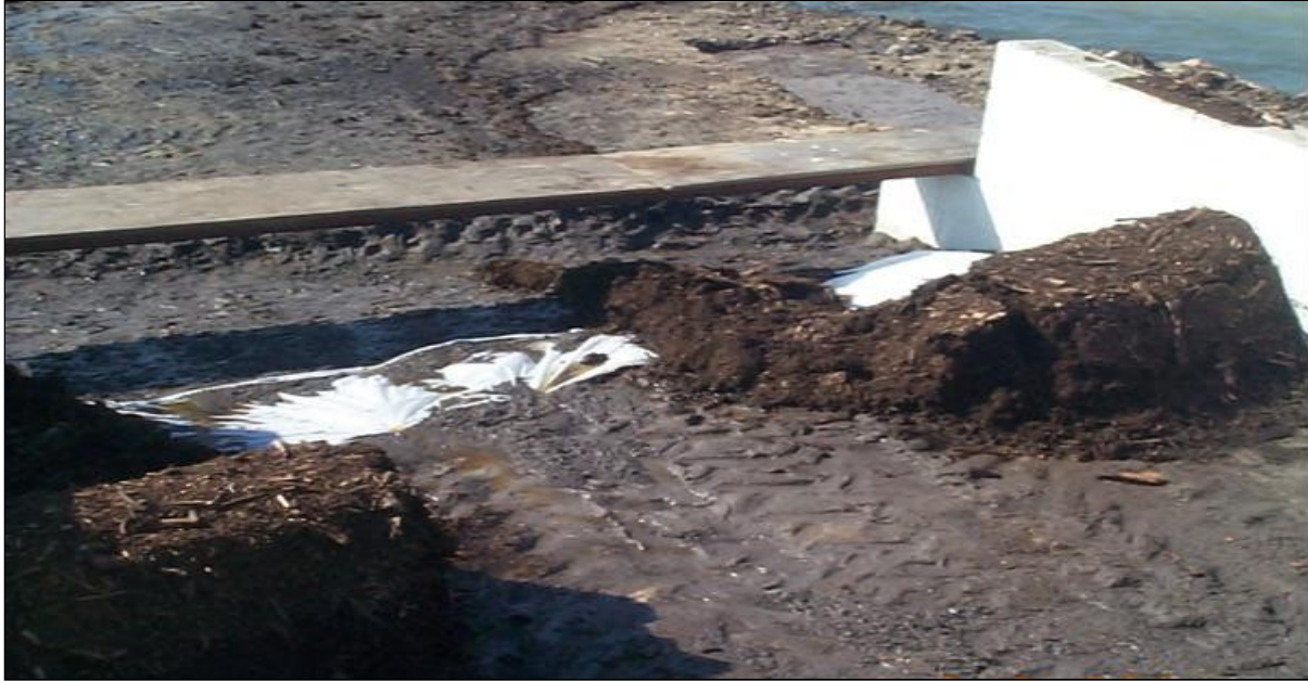
Figure 4.3. No Traction between Clay Soil and CBS Berm Leading to Displacement of Berm.
