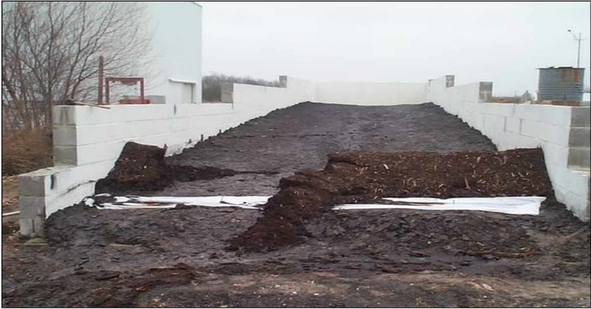
Figure 4.1. Failure of the DMC Berm on Clay Due to Displacement (Round 1-1).
