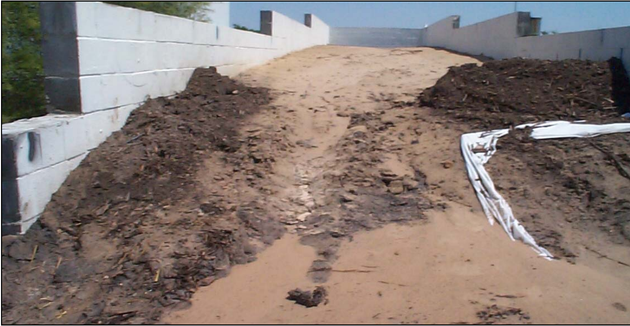
Figure 4.7. Failure of CBS Berm on Sand.
