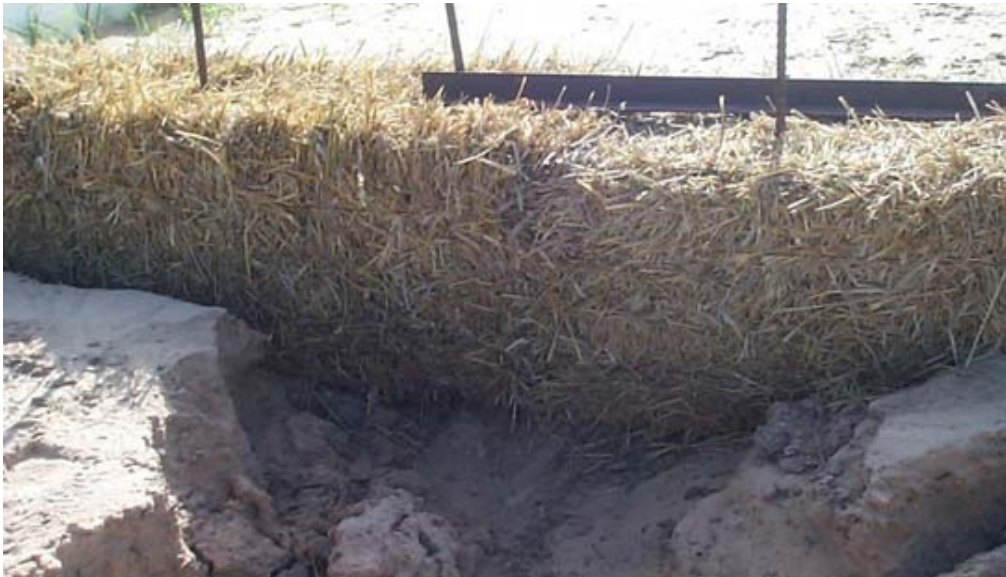
Figure 4.15. Scouring Downstream of the Straw Bales.
