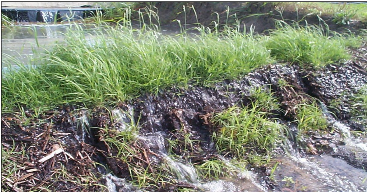
Figure 4.12. Dairy Manure Compost Berm Showing Minor Damages to the Leading Face.
