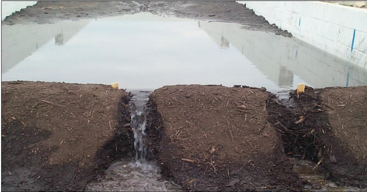
Figure 4.5. Failure around the Stakes When the Berm Was Anchored.
