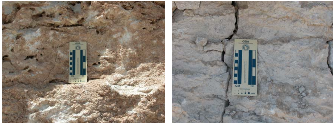
Figure 6. Image on Left Shows Vugs in the Limestone, and Image on the Right Shows Stylolites That Contain Clay Minerals.
