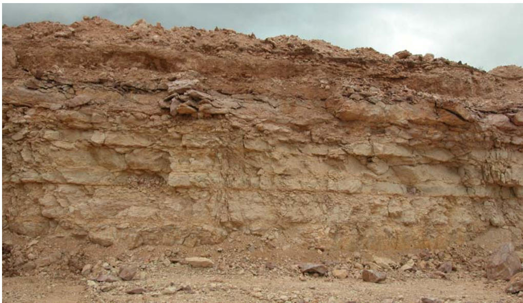
Figure 8. Working Face at the Clements Pit Showing Thin, Laterally Extensive Limestone Beds.
