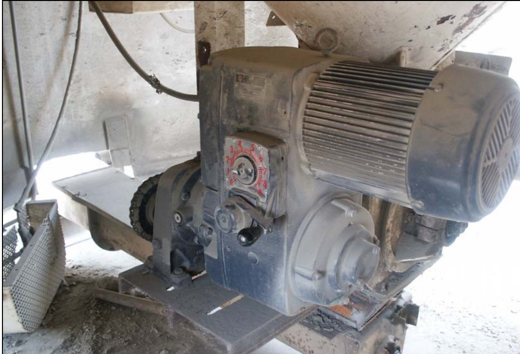
(a) Meter for Adjusting Amount of Cement Pumped to the Pugmill.
