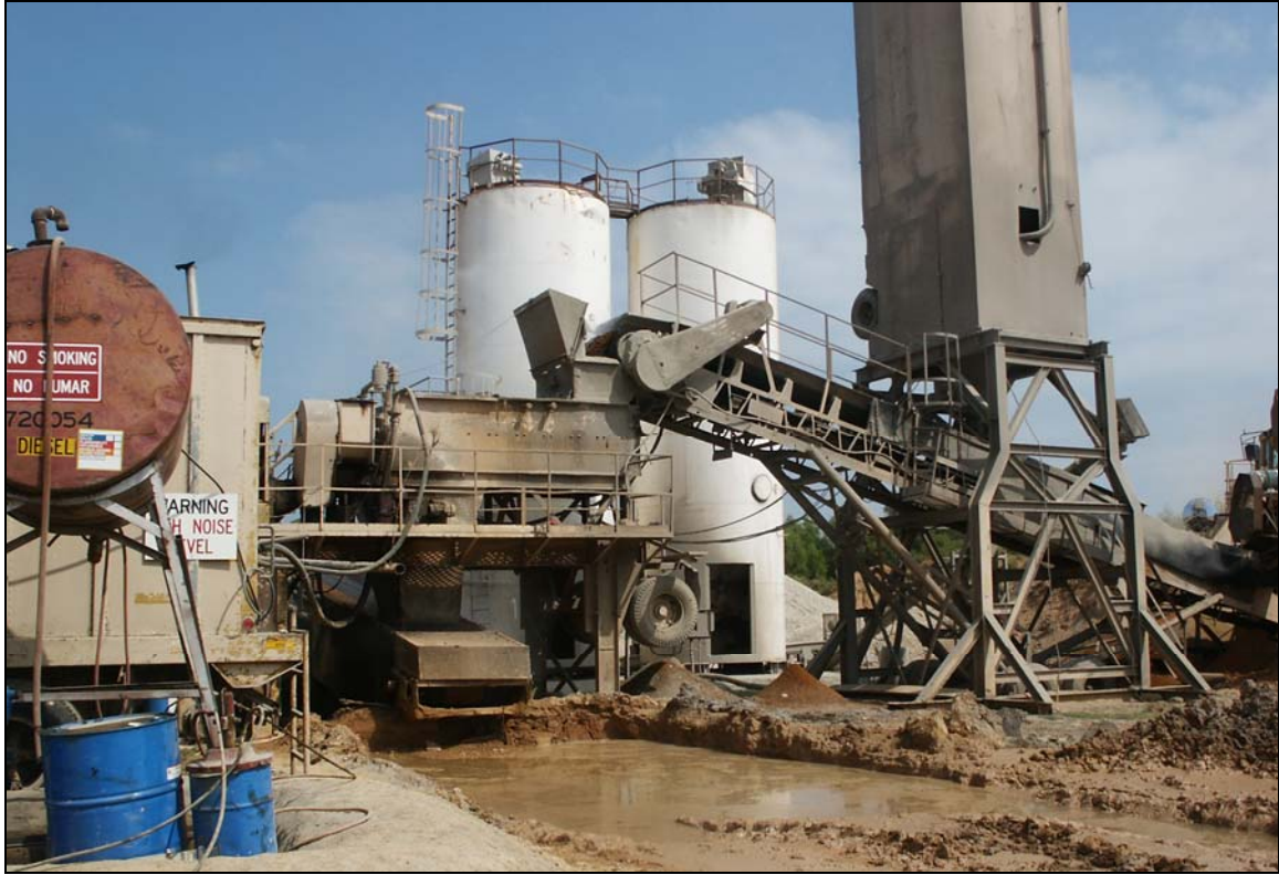
Figure 4.16. Scarmardo Pugmill Mixing Plant.
