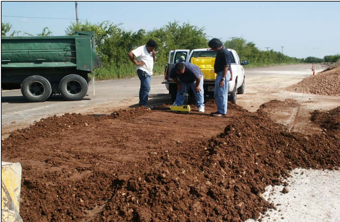
Figure 4.5. Checking Moisture Content of Base with Nuclear Gauge during the Mixing Process to Target Optimum Moisture Condition.
