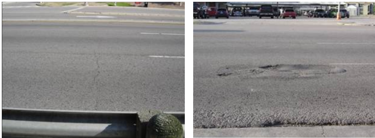
Figure 2. Photograph of Distresses on Loop 12.
