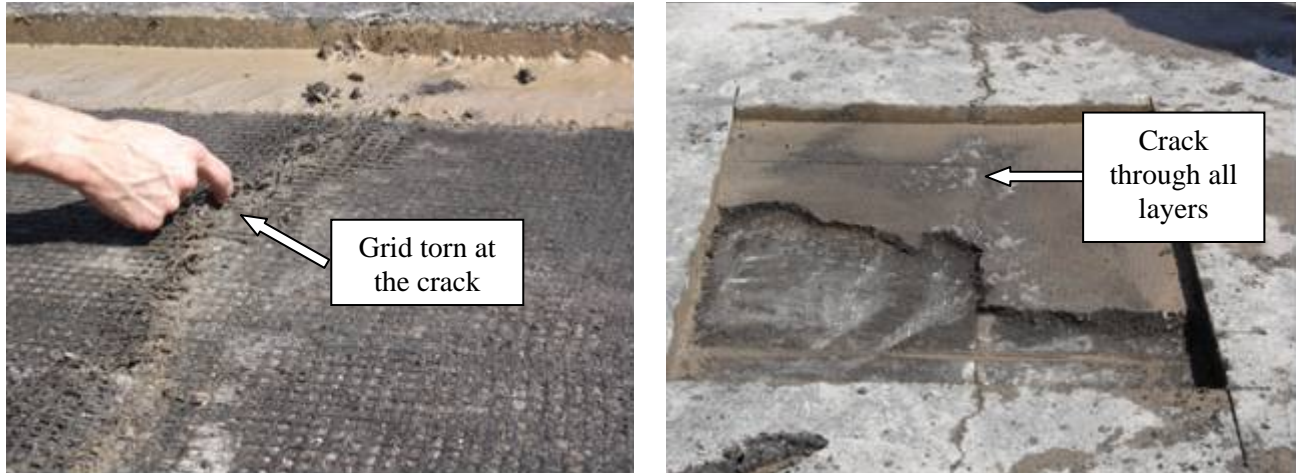
Figure 4. Photographs of a Trench at a Transverse Crack on Loop 12.
