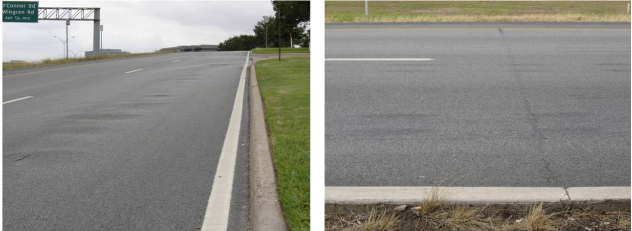
Figure 26. Photographs of Shoving and Transverse Cracks on SH 114.
