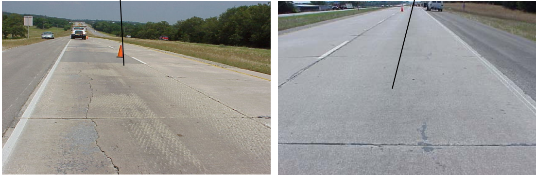
b) Pavement Condition in the Distressed and Non-distressed Area
