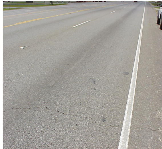
d) Control Section Regular Transverse Cracking
