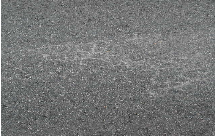
Figure 34. Initial Indications of Problems on GlasGrid® Installation on IH 45 in the Bryan District.
