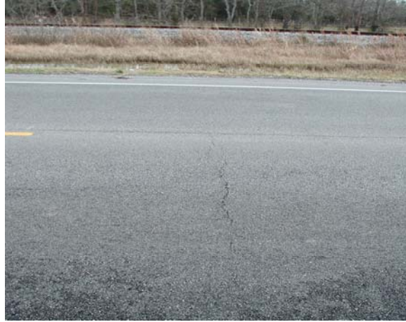
Figure 21. Reflection Cracks in the Control Section after One Year.
