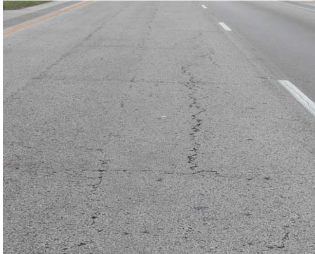
Figure 6. Condition of Section R4 in 2003.
