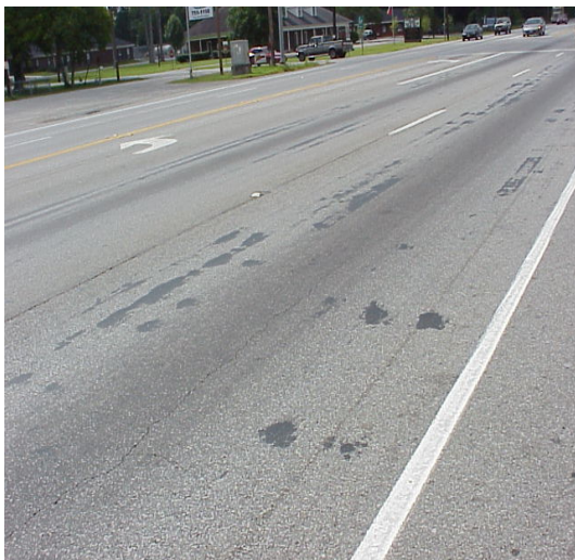
c) GlasGrid® Significant Longitudinal Cracking and Some Transverse
