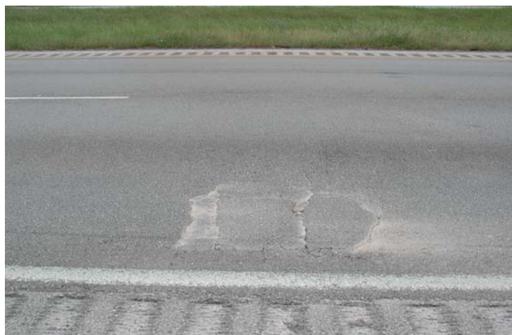
Figure 4. Continued Failures in Section 2B the Crack and Seat Section after Multiple Repairs.
