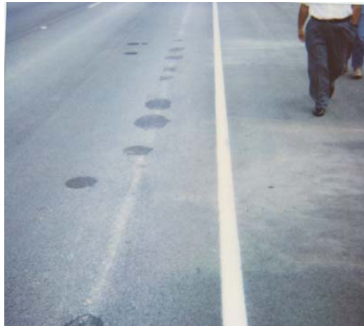
Figure 32. Failure of the GlasGrid® Section on IH 45, Houston District (1999).
