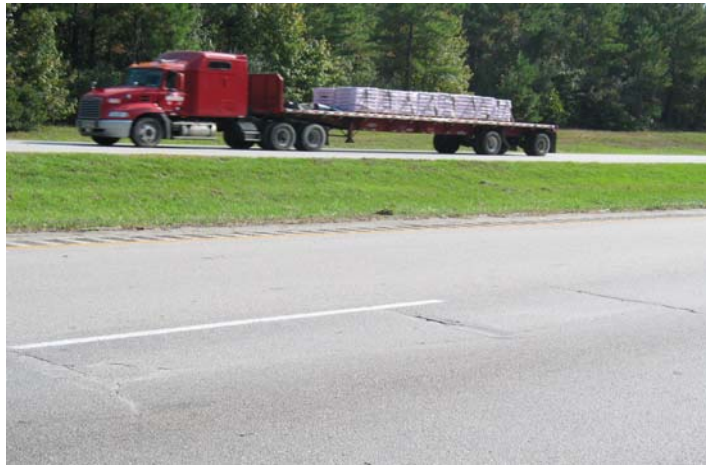
Figure 3. Section R1 in 2003, Additional Patching with Reflection Cracking.
