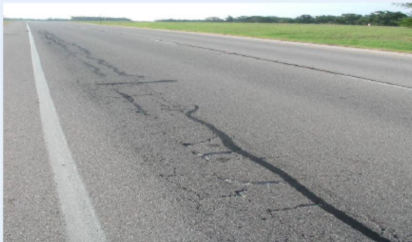
Figure 1. Alligator Cracking in the Wheel Path of SH 47
