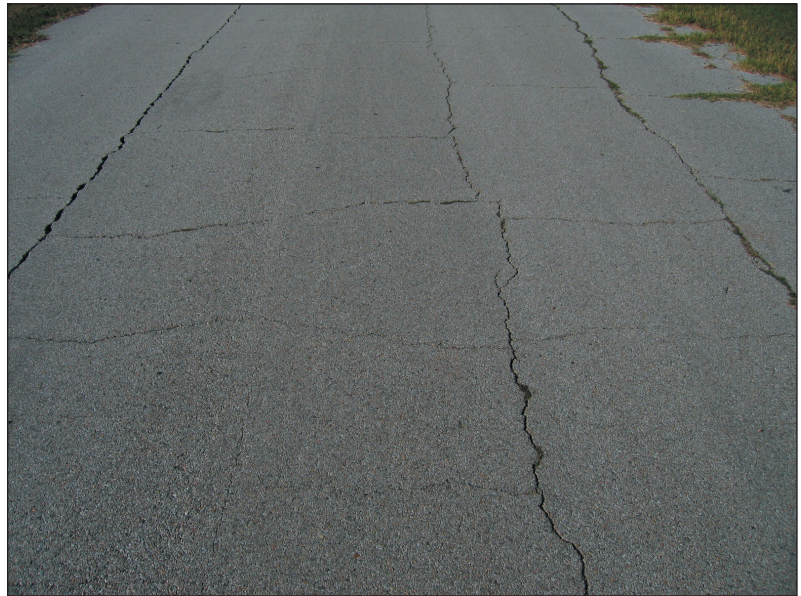
Figure 1. Shrinkage Cracking Resulting from Problems with Cement-Treated Base.
