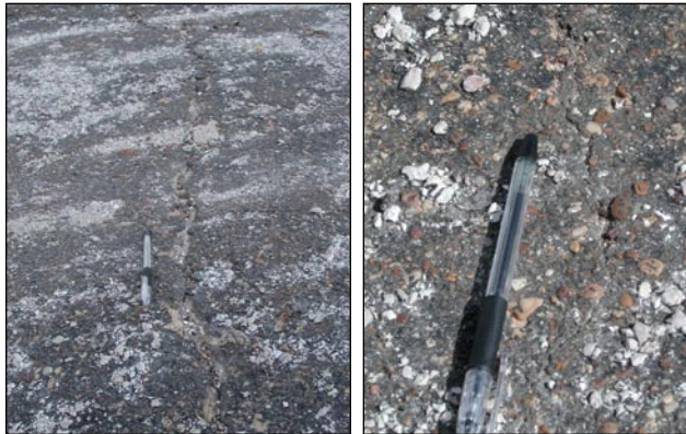
Crack in moist-cured section.
