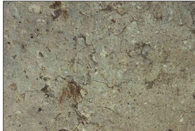
Visible cracks in CTB after microcracking are rarely observed.
